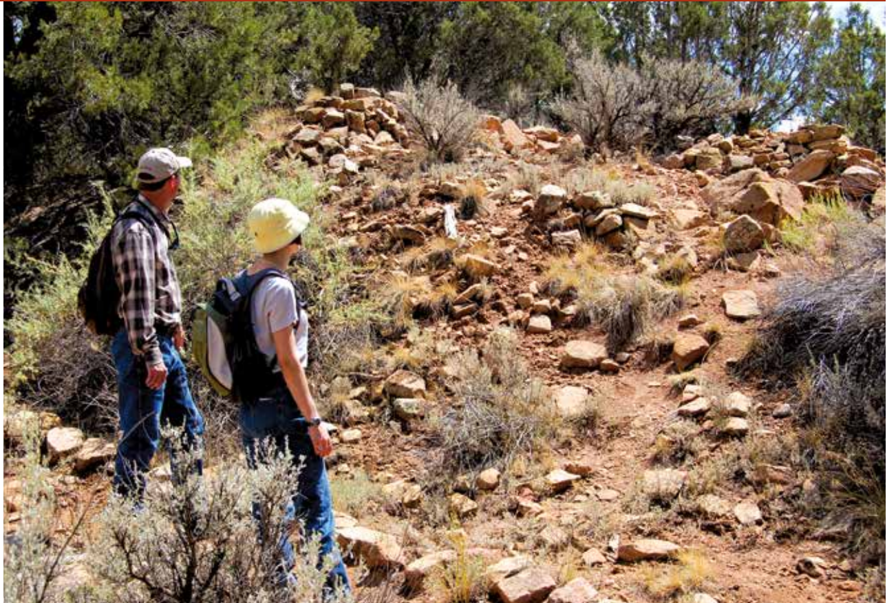
Sand Canyon Pueblo was occupied at the same time as Cliff Palace at Mesa Verde National Park. An open site with no protection from the weather, Sand Canyon Pueblo's ancient walls have collapsed.
