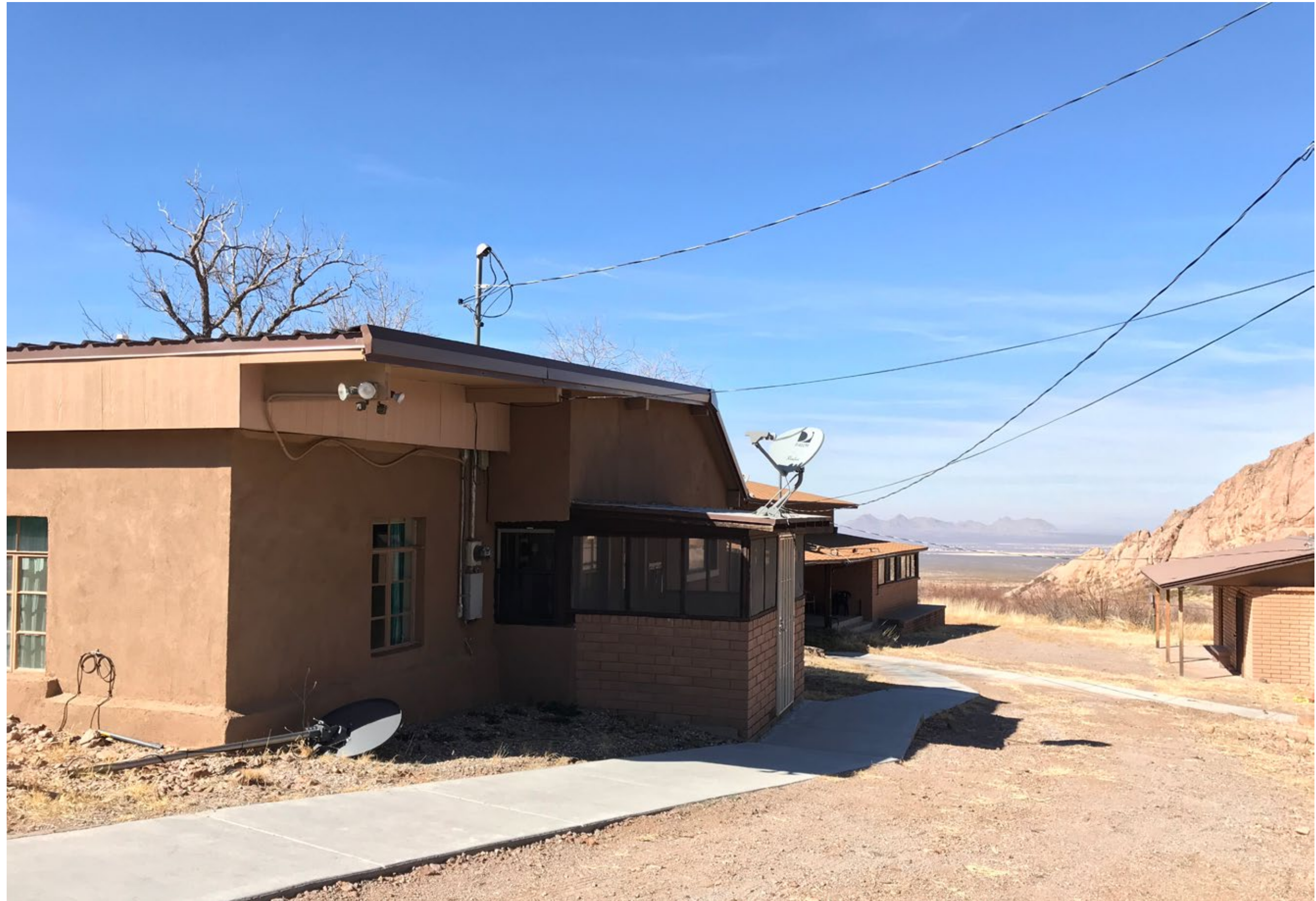
Slide 26 is a photo of the back of the house, immediately east of the Cox Visitor Center. It indicates that the house has been remodeled (and perhaps not sensitively) on multiple occasions.
