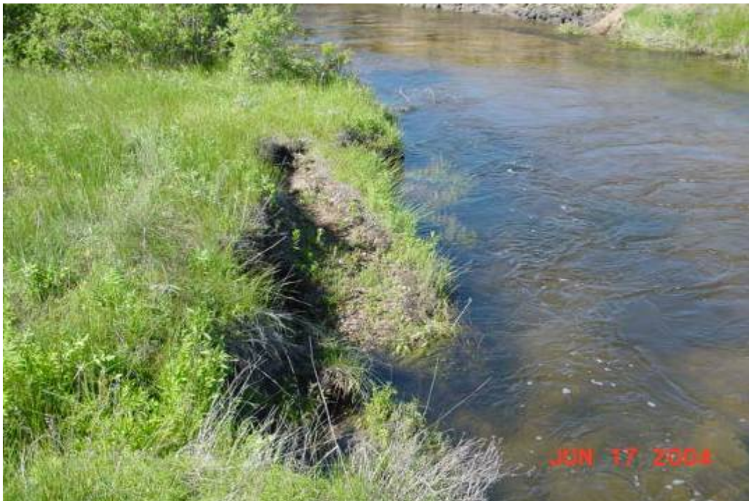
Figure 4 —the photo above shows a fracture and a large slump that is still attached to the streambank. Vegetation cover is at least 50 percent canopy cover and is classified as covered/unstable (CU). (see Illustration 4)
