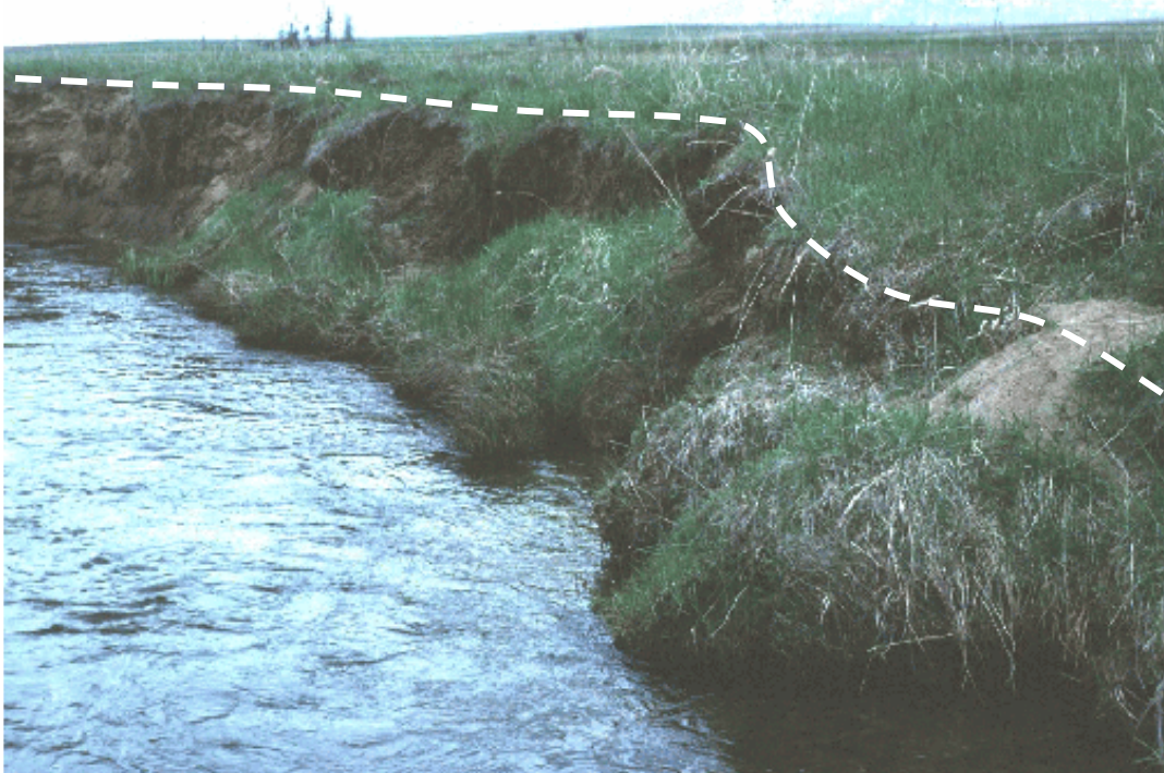
Figure 32 —slump block detached from the streambank and not stabilized with vegetation.
