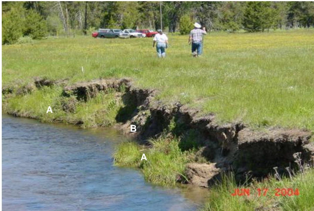
Figure 5 —the stream in this photo is flowing at the scour line. Slumps “A” are still attached the bank above the scour line and would be classified as covered/unstable (CU) (See Illustration 4). “B” has no vegetation along the streambank and is uncovered/unstable (UU) (See Illustration 4).
