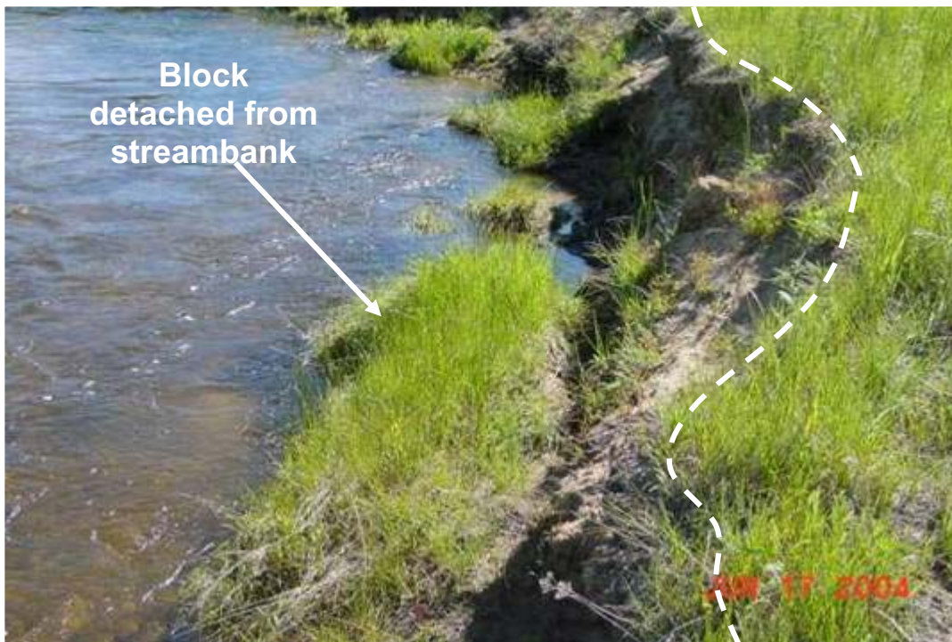
Figure 30 —slump block detached from the terrace wall. There is still a high potential for erosion between the slump block and the terrace wall.
