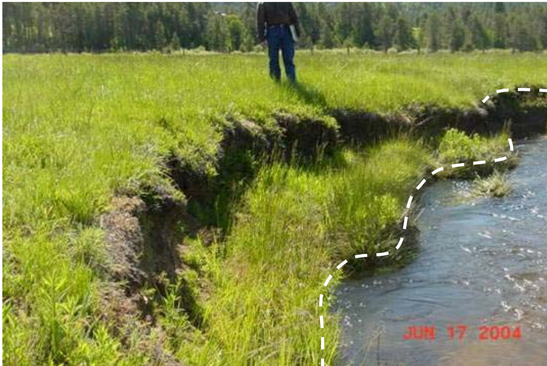
Figure 29 —slump blocks vegetated to the terrace wall. New floodplain is being established. The vertical walls will continue to erode until they reach the angle of repose and revegetate.
