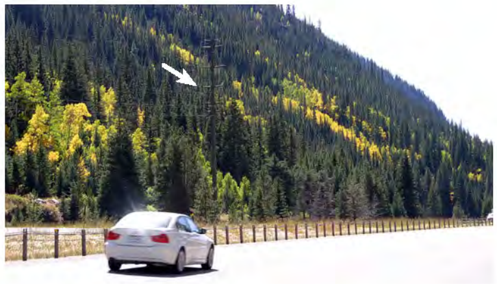
Transmission power line that was factory painted with a single color and installed circa 1976.
