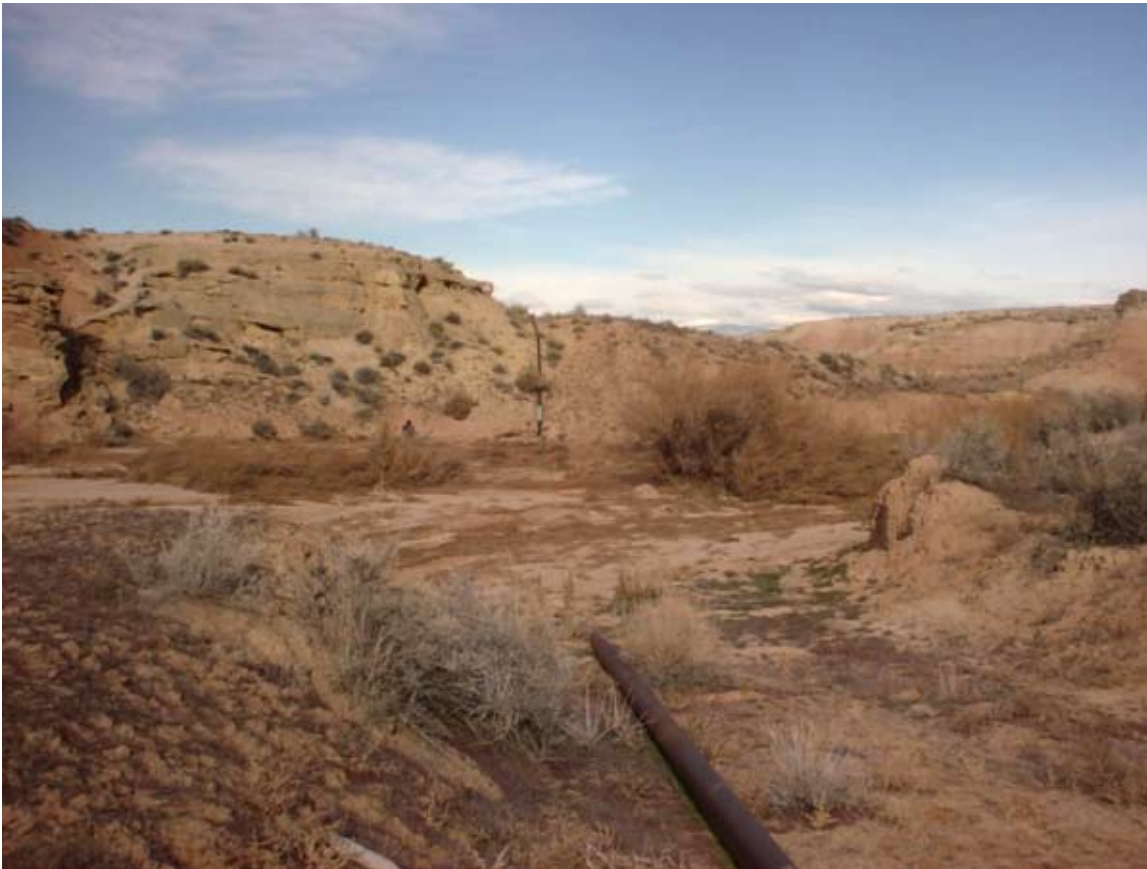
Figure 6. Channel degradation or scour during flash-flood events may expose buried pipelines, resulting in costly breaks.
