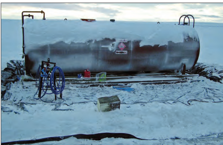
Figure 22. Containment around a bulk fuel tank at a remote O&G support camp.
