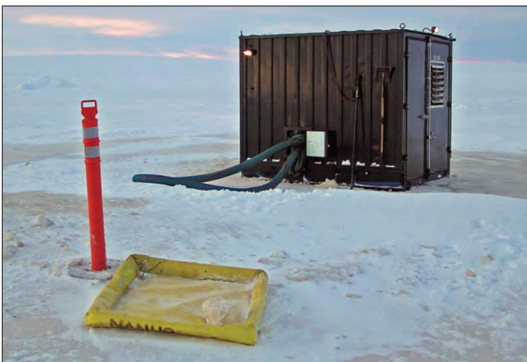
Figure 21. Portable drip pan for water trucks that fill up on a water source lake.
