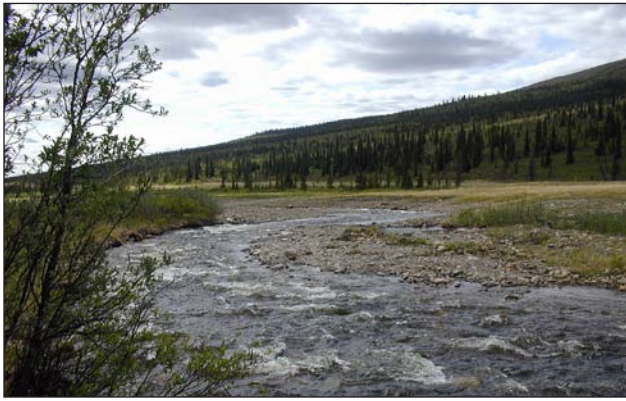
Figure 12. In the upper reclamation area, the meanders had to be increased and the point bars leveled to stabilize the channel. Note the grass in the background, a result of hydroseeding during road construction.
