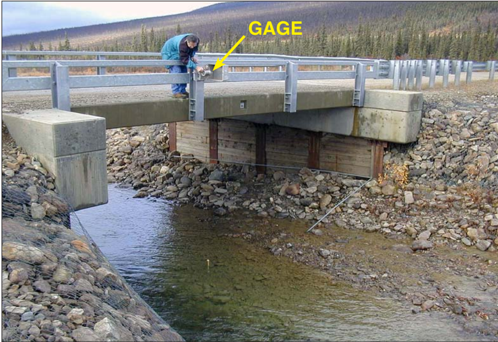
Figure A-3. Looking downstream at the wire-weight gage reach for Nome Creek at the bridge. The gage was installed in 1998 on the downstream side and relocated to the upstream side of the bridge in 1999. Gaging continues to the present.
