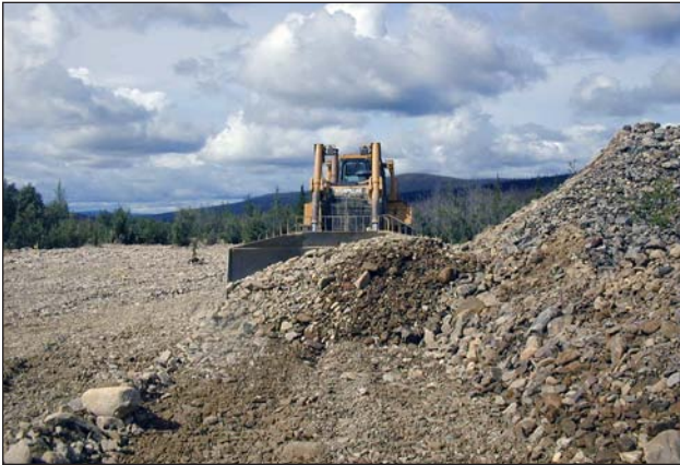
Figure 6. After filling the ponds, the bulldozer then graded the floodplain as flat as possible.
