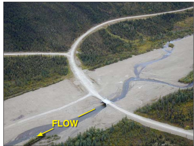
Figure 9. Aerial view of the channel upstream of the bridge, where the gabions are being eroded by the unstable channel.
