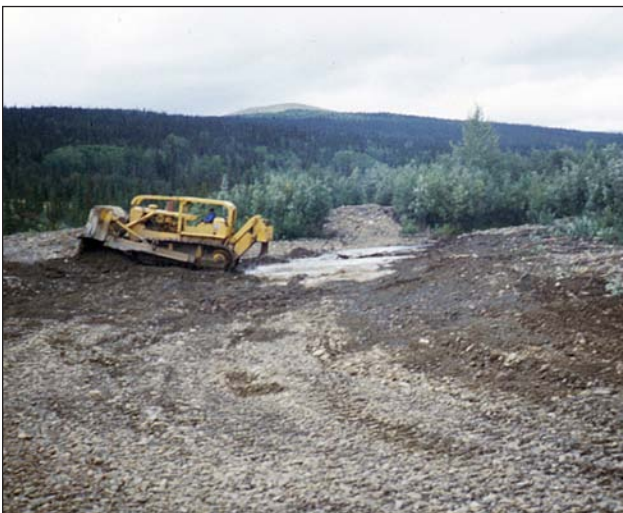
Figure 7. The bulldozer constructed the channel using short, almost level grading to deepen the pilot channel.
