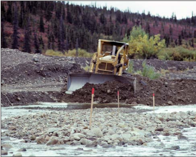
Figure 5. The initial step in reclamation was to fill the settling ponds with the dozer, using the material from the surrounding tailings piles.
