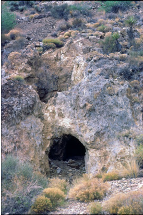
Figure 3.11. Unreinforced adit portal, C&K Mine, Providence Mountains State Recreation Area, San Bernardino County, 1989 (photograph by Karen K. Swope).
