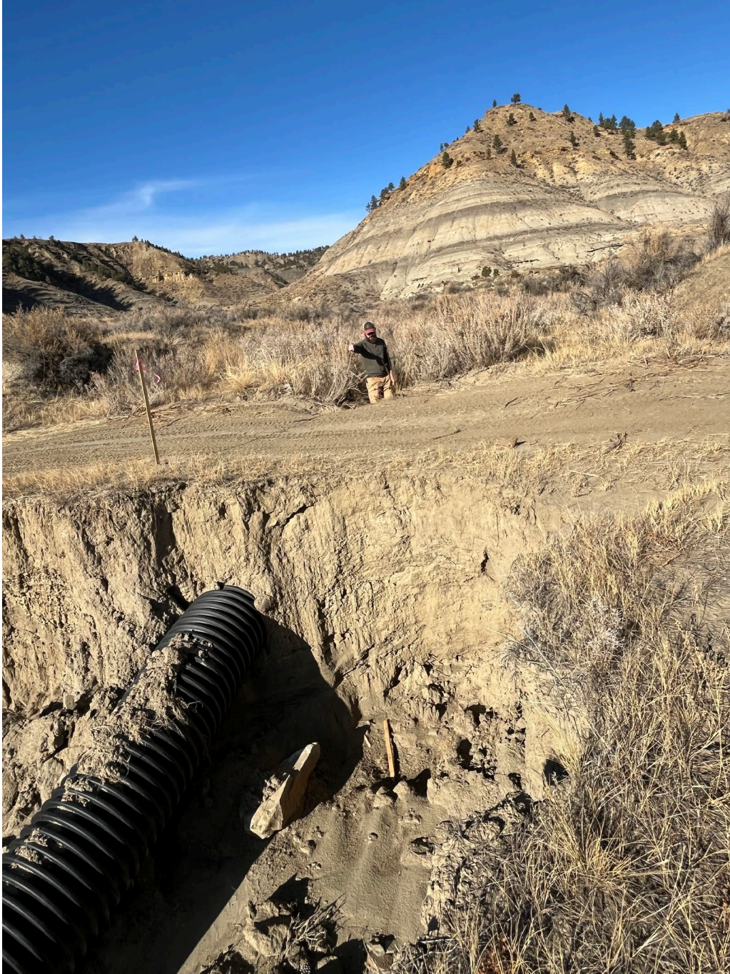
Figure 2: BLM employee showing erosion conditions from a failing culvert
