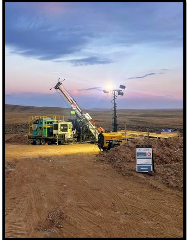
Figure 6: Photograph of an active drill site. The site perimeter is clearly defined with subsoil berms and signage to prevent unauthorized entry and contain the drill site area.
