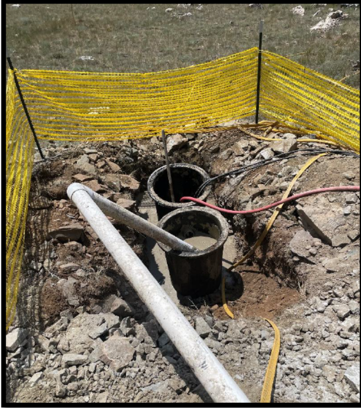
Figure 5: Photograph of a sump at an active drill site. Note the containment buckets for drill cuttings and water recirculation through hoses for water recycling during the drilling process. High-visibility safety fencing is temporarily installed while the sump is in use to prevent any unauthorized entry and contain the sump area.
