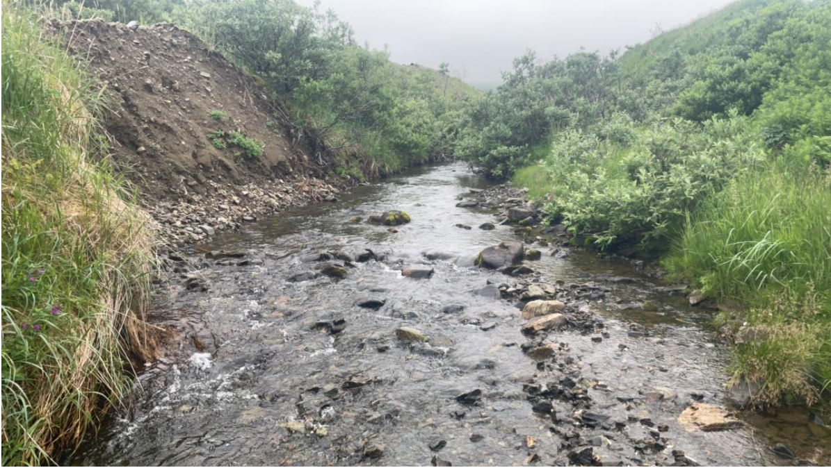
Photograph 13. Downstream view of Platinum Creek showing a confined section with no floodplain and bank erosion.
