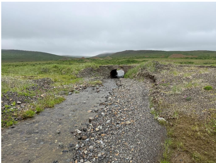
Photograph 5. Undersized culvert on Dowry Creek (downstream view). Note enlarged channel and sediment deposition upstream of culvert.
