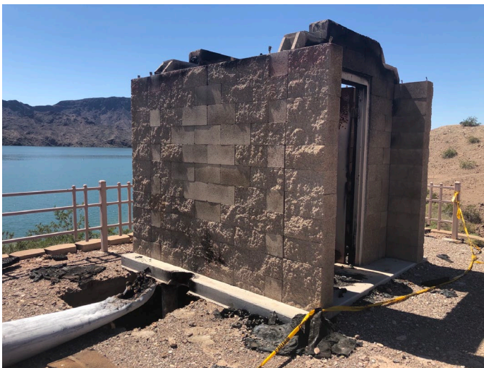
Vandalized Vault Toilet
