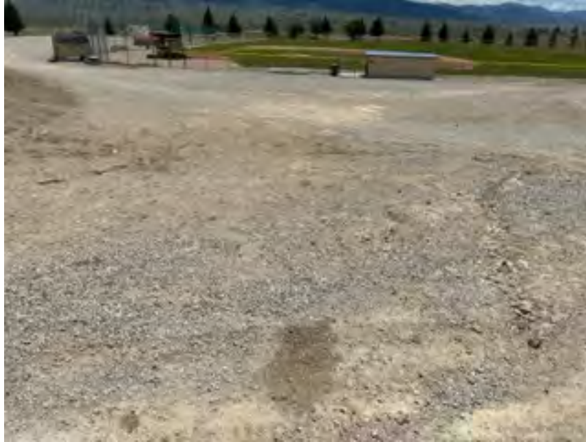
Photo 5: Ely Little League Fields Renovation- Uneven hill from parking to field 3, looking southeast
