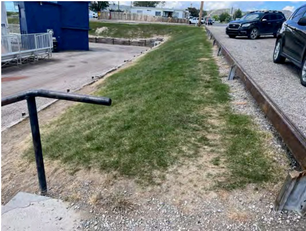
Photo 2: Ely Little League Fields Renovation Northwest Corner Retaining Wall, Field 1 Press box, StreetSide Parking, Stairs to Fields, looking West
