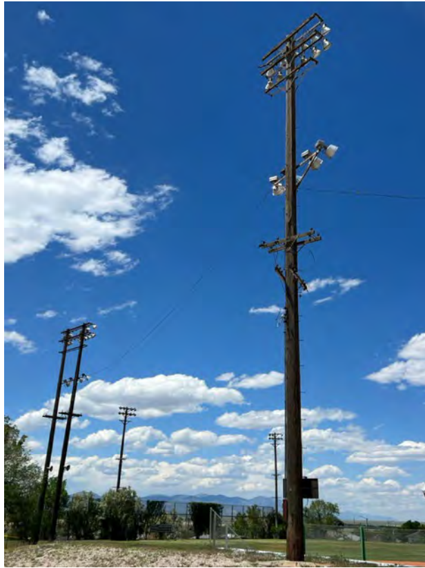
Photo 1: Ballfield Overhead Light Poles
