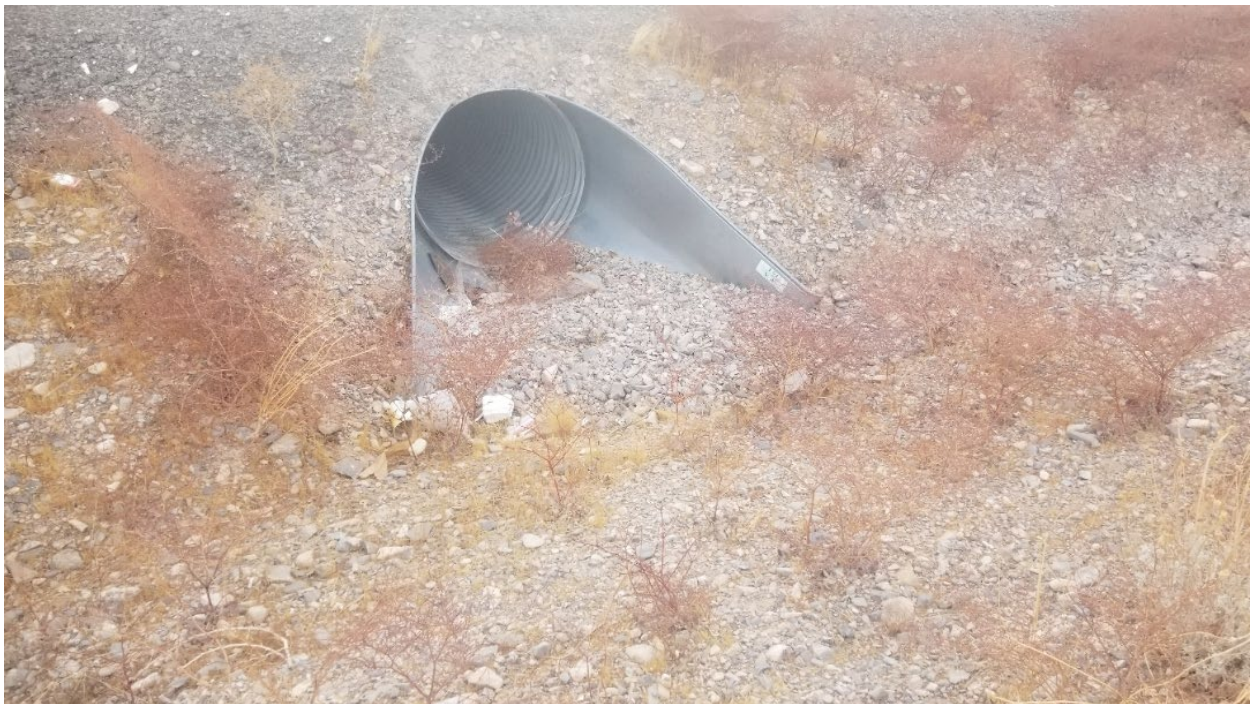
Photo 2. Corrugated metal culvert with no fencing attached.
