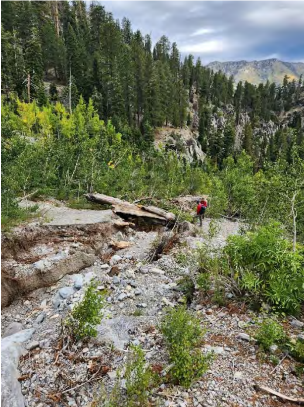
Photo 4: Significant trail damage (complete loss of trailway) at trail mile 0.9.
