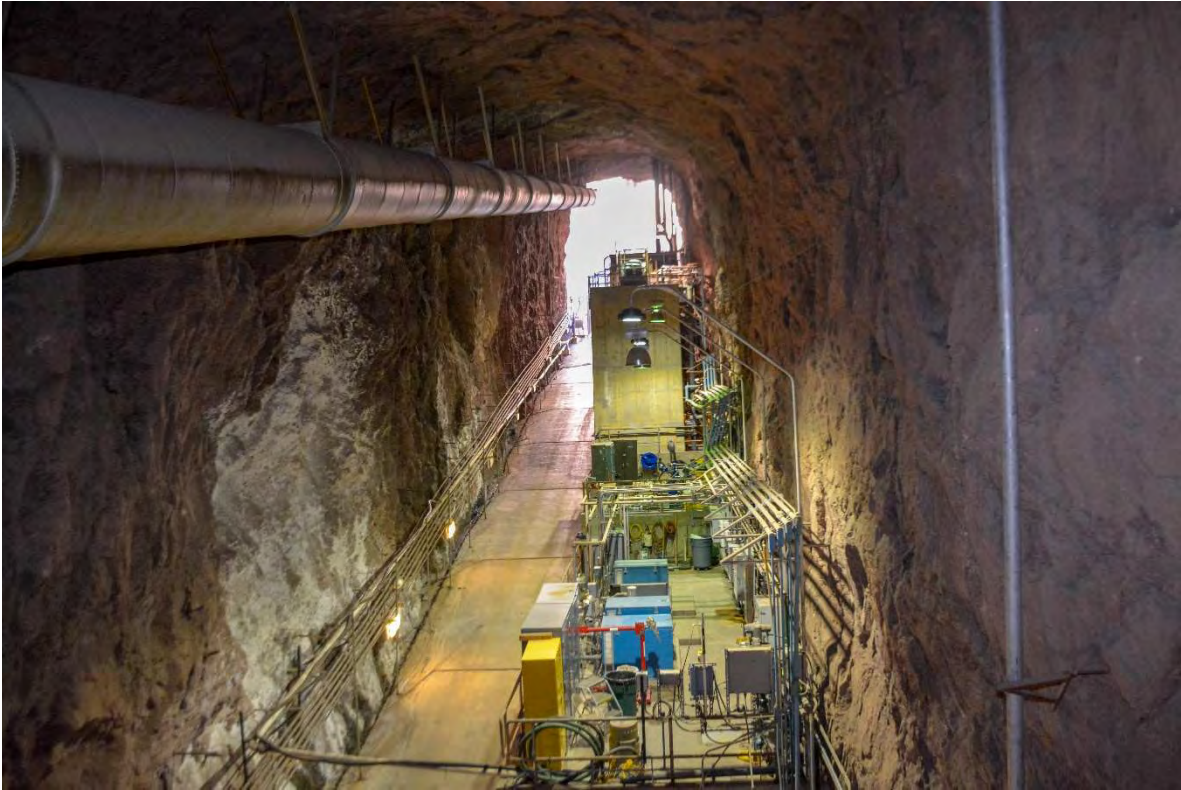
View from penstock platform of existing Wastewater Treatment plant located in Arizona penstock access tunnel showing no room for expansion.
