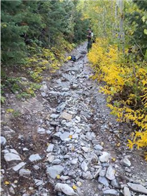
Photo 1: Typical trail damage between trail mile 0.2 and 0.9.
