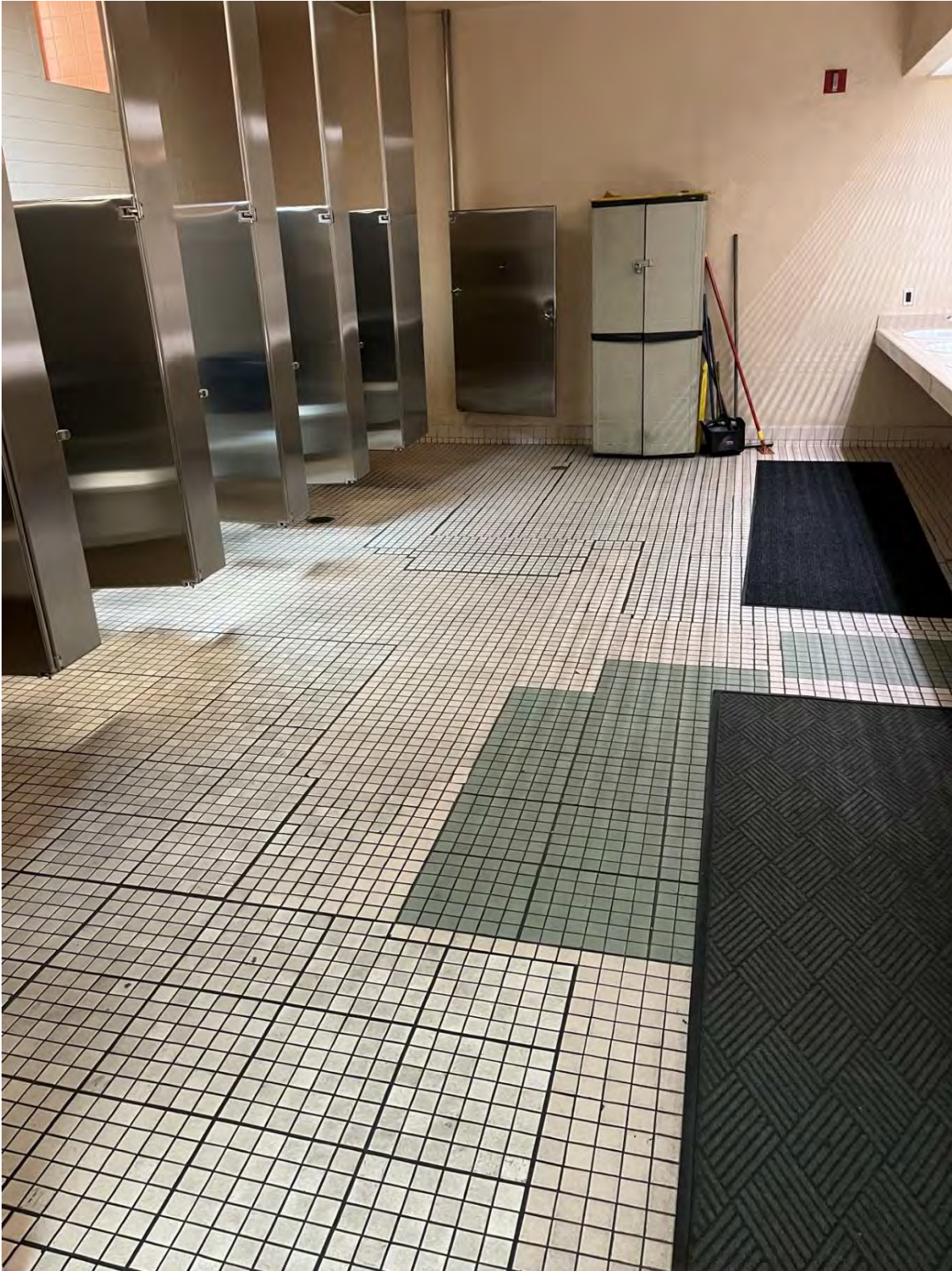
Parking garage restroom showing deteriorated condition and need for major renovation
