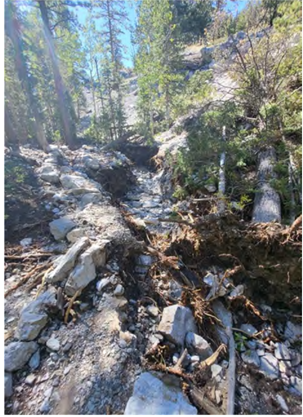
Photo 2: Typical example of severe rutting along trailway on upper portion of the trail.
