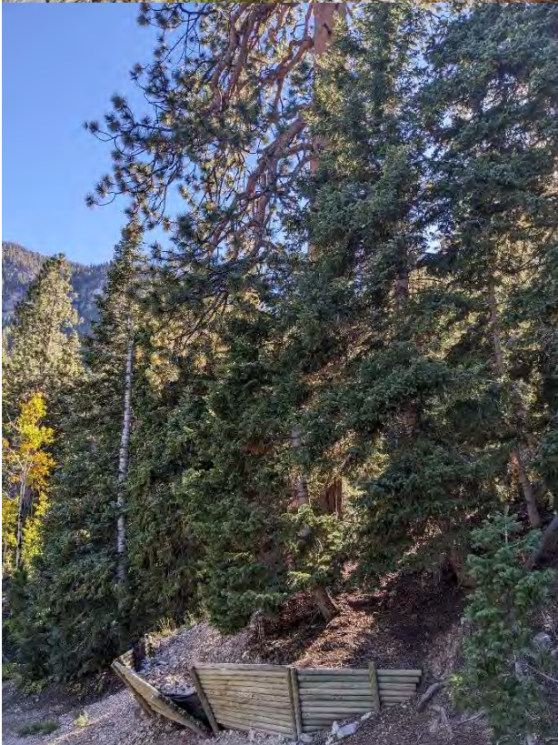
Photo 5: Failing retaining wall along trail at approximately trail mile 1.0.
