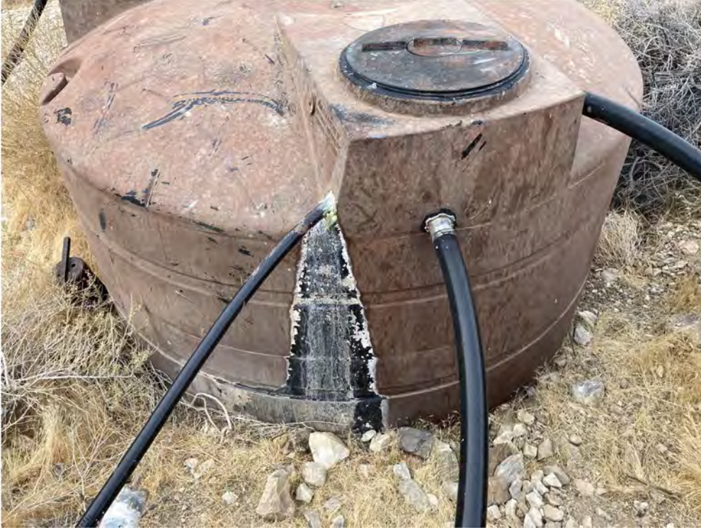
Figure 4: Degraded storage tank and plumbing
