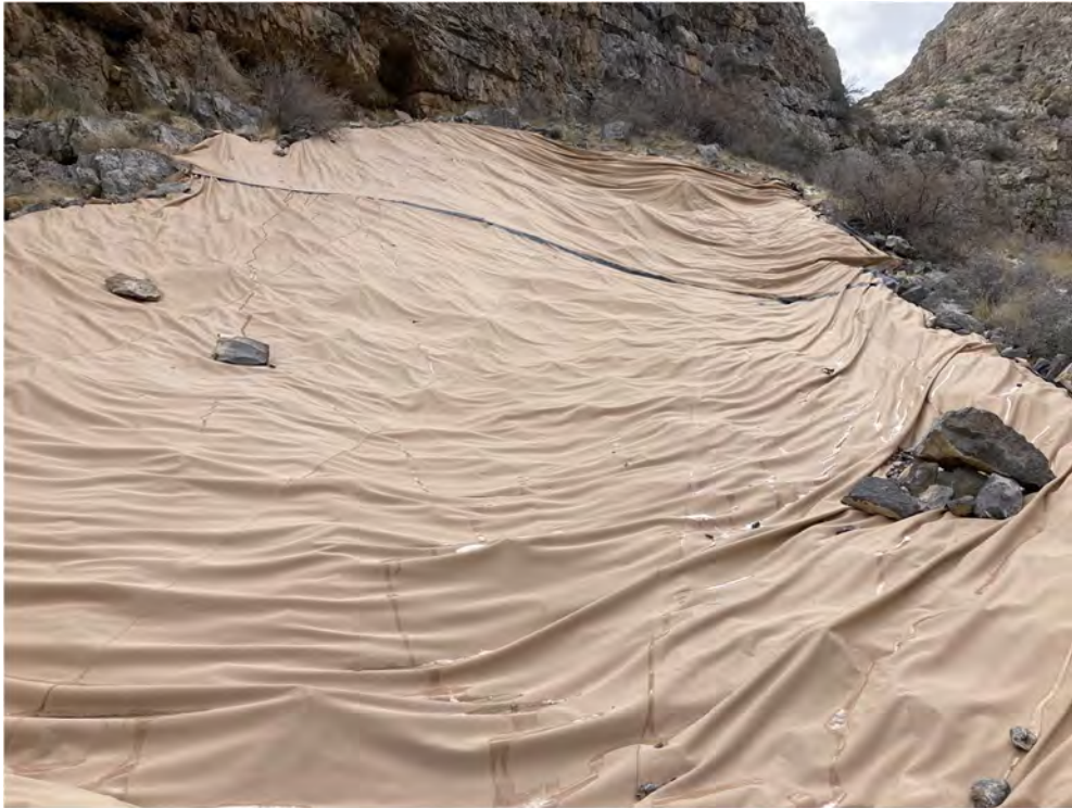
Figure 3: Degraded and cracking old hyperlon apron
