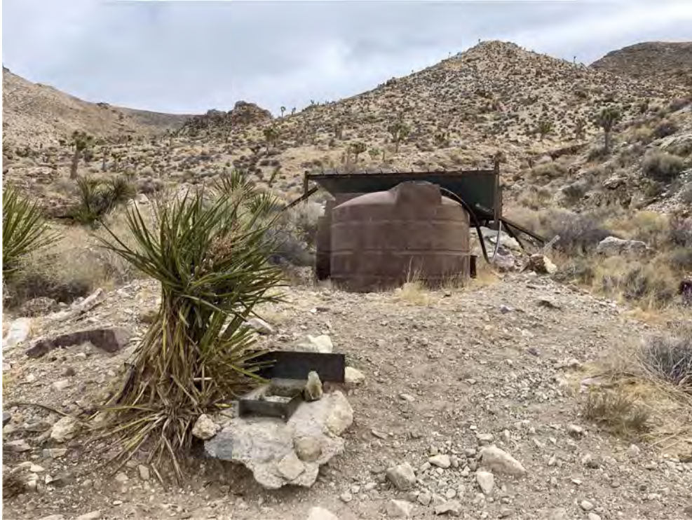
Figure 2: Mostly dysfunctional Quartz Spring hybrid system with old storage, empty float valve drinker, small apron and non-functioning connection to spring
