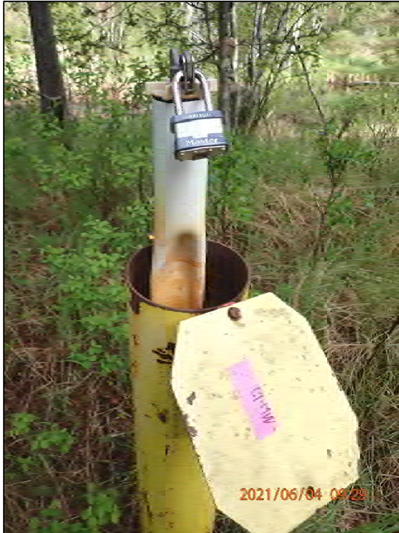
Photograph 2-2. MW12, frost jacked with collapsed PVC. June 4, 2021.
