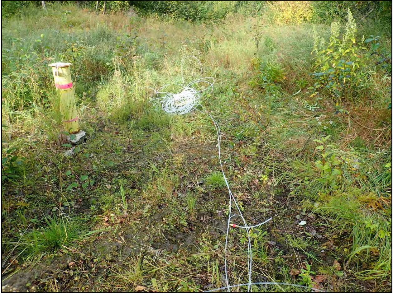
Photograph 2-24. MW59 damaged tubing after removal. September 1, 2021.
