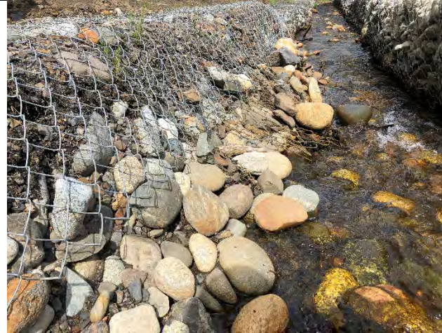
Date: 6/23/2020 Direction: NE Description: Damaged gabions as part of drainage and NTCRA.
