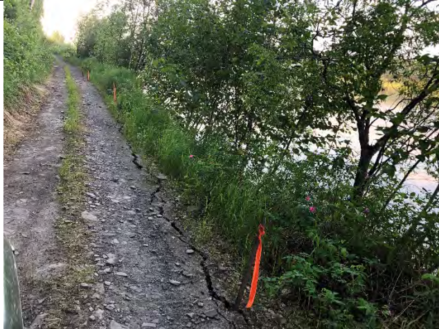
Date: 6/16/2020 Direction: NW Description: Tension cracks along service road to RDM.
