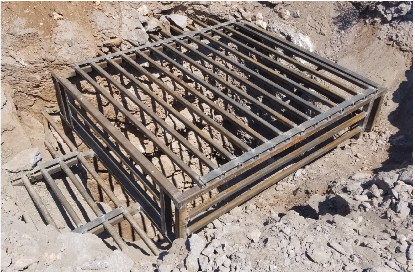
A remediated mine shaft to address human health and safety from BIL Phase 2
