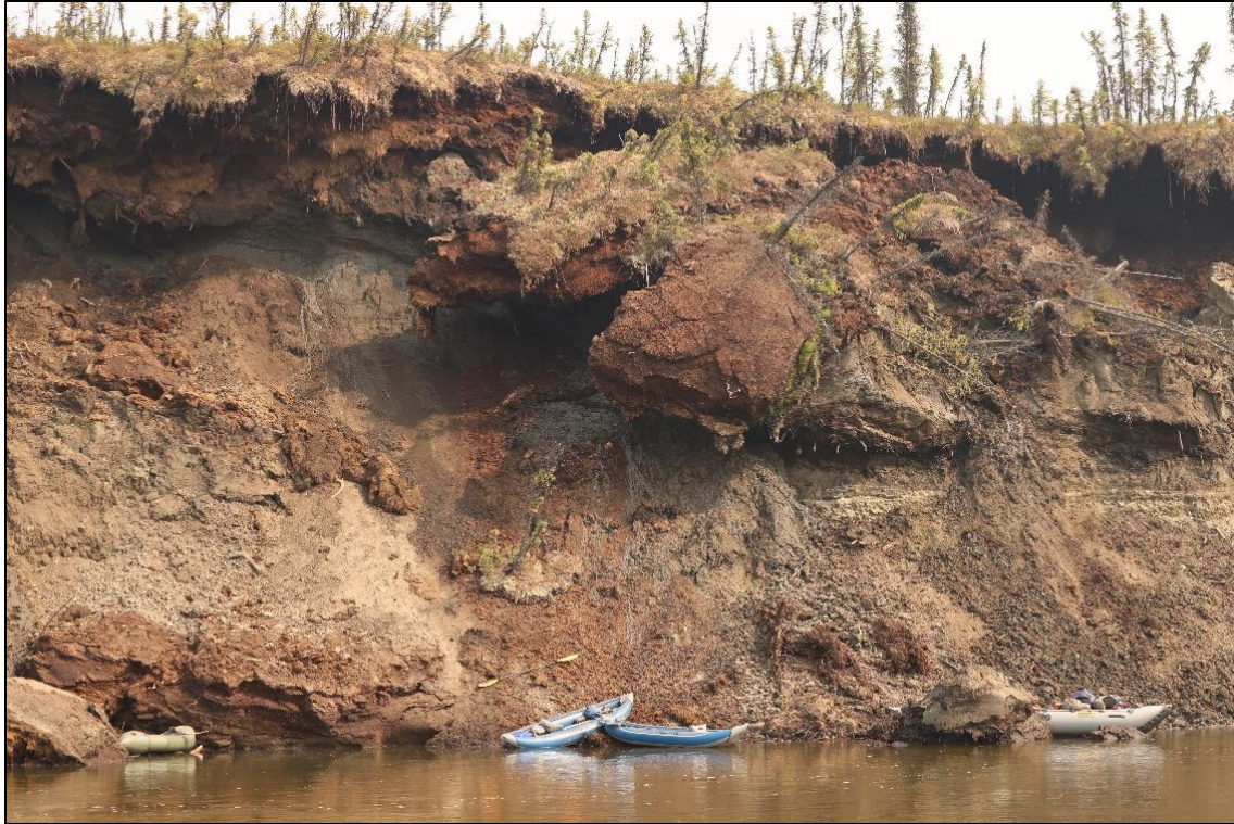
Figure 6. Streamside photograph showing unstable embankment, melting permafrost area, lower Birch Creek WSR, June 2022.
