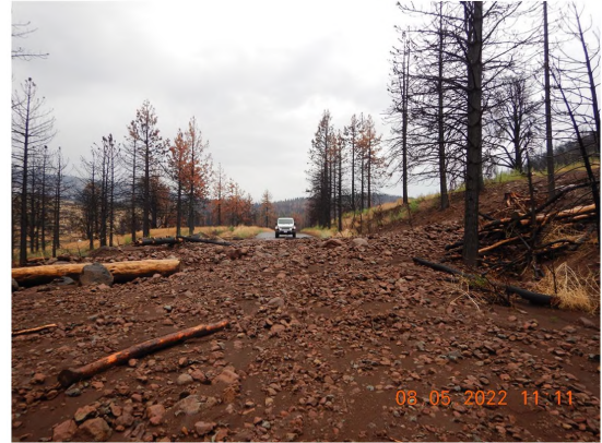
Campground Road Washout.
