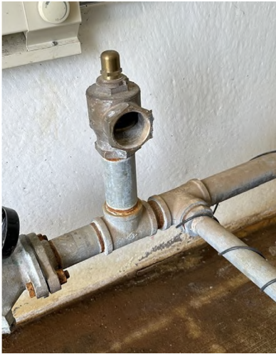
Replace relief pressure valve with a screened one.
