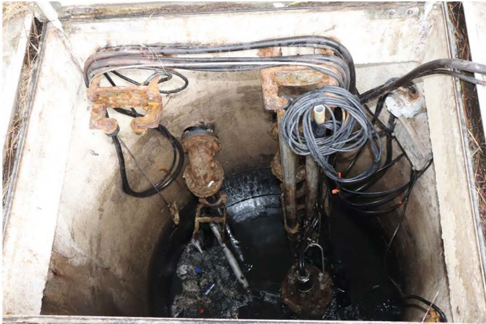
Aging Lift Station at Pink House
