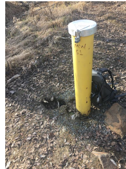
Photo 4: Soil settling in the vicinity of MW51.
