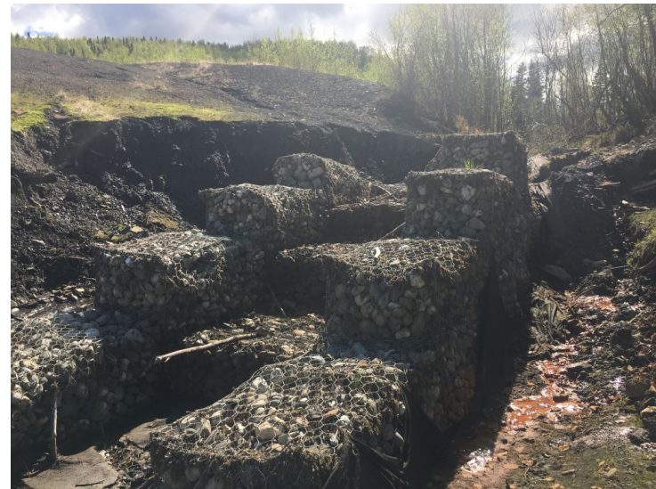
Photo 16: View from left bank of Red Devil Creek to upstream NTCRA gabions. New seep visible in right of photo.
