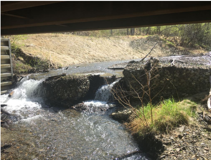
Photo 13: View upstream from left bank of Red Devil Creek to breached gabions of sediment settling pond.
