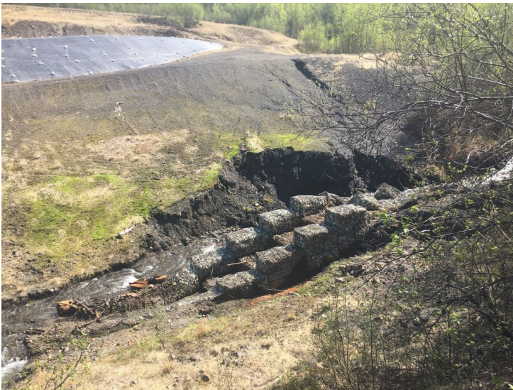
Photo 15: View from pre-1955 MPA to breached NTCRA gabions.
