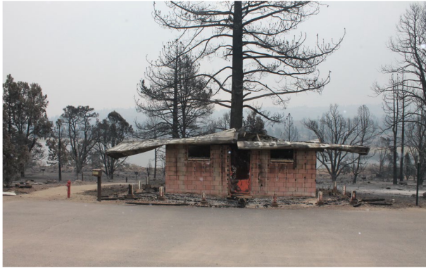
Destroyed bathroom at Indian Creek Campground
