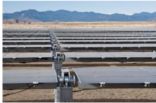
Typical Tracker Array Configuration and Mounting Systems
