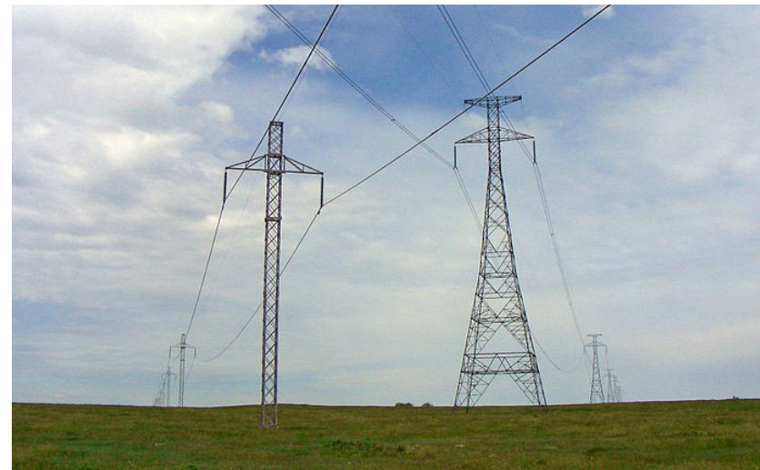
Figure 5-2. High Voltage DC Structures
