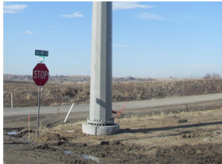
Figure 5-18. Single-pole Steel Structure on Concrete Pier Foundations
