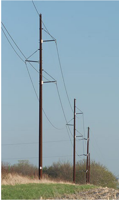
Figure 5-4. Single-pole Wood Tangent
