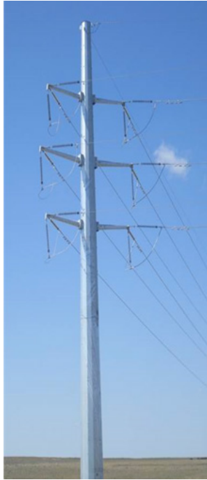
Figure 5-5. Single-pole Steel Dead-end
