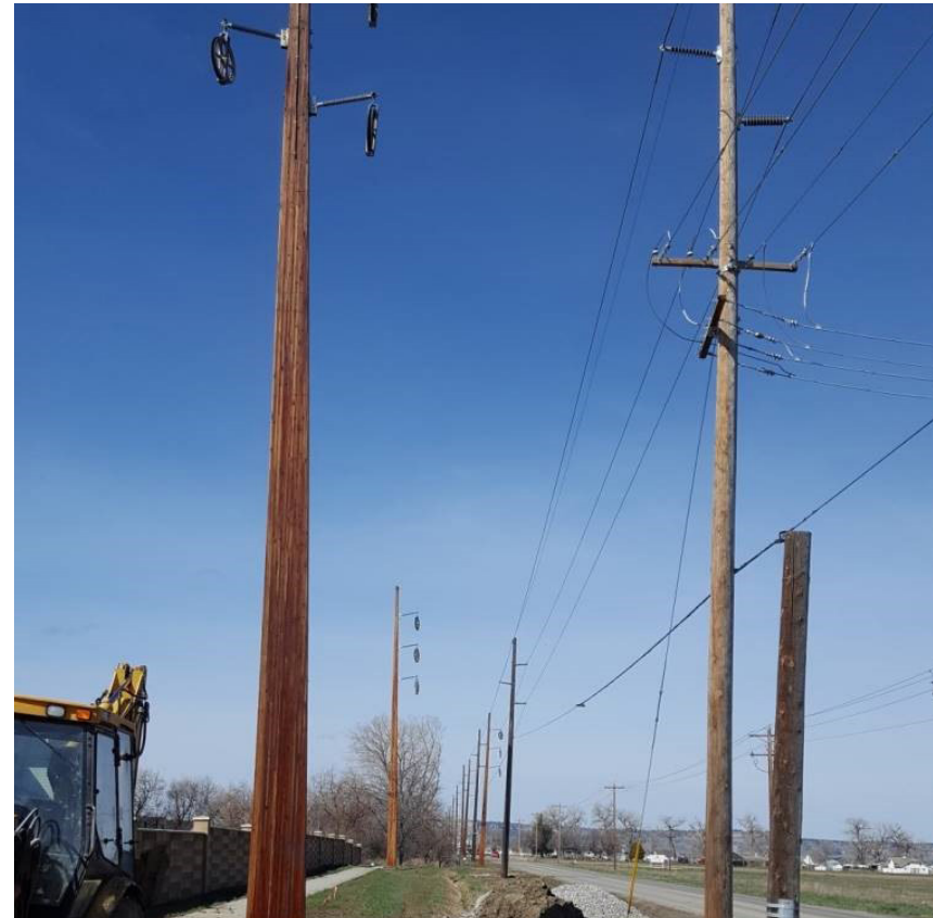
Figure 5-9. 100 kV Laminated Wood Pole (left) Typical Wood Pole with Guy (right)
