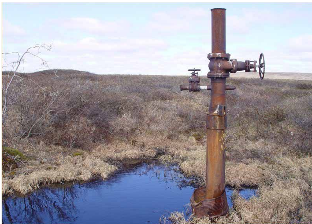
Figure 4: Umiat #10 prior to plugging operations (June 2003).
