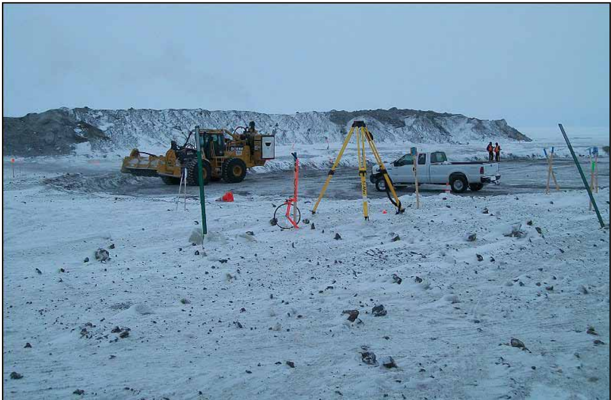
Figure 9: Excavation of the reserve pit at Drew Point #1 occurred concurrently with the well plugging operations (March 2010).
