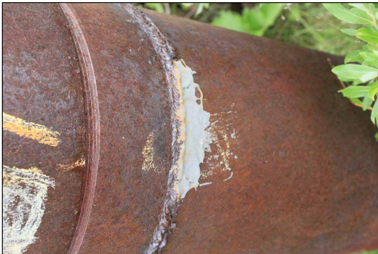
Figure 4: Wolf Creek #1 close-up of the J-B Weld patch (July 2012).
