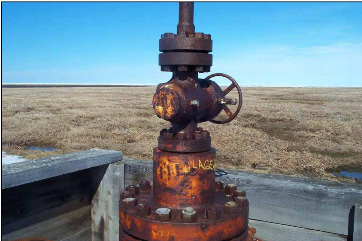
Figure 10: Gate valve on Tulageak #1 (June 2003).
