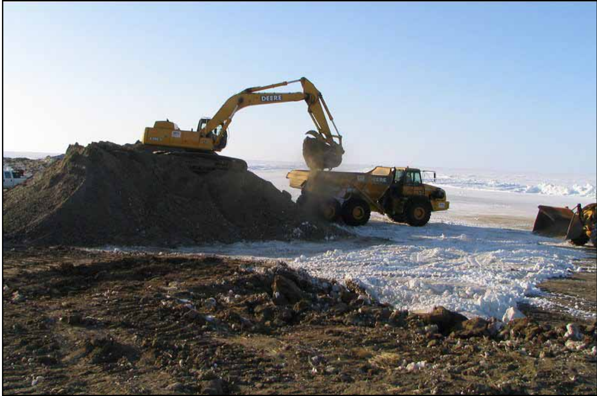
Figure 9: Diesel-contaminated soils are loaded into a dump truck, which transported the material by ice road to the North Kalikpik well site reserve pit (April 2008).
