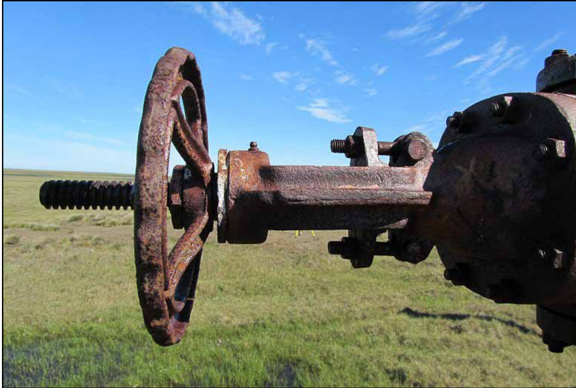
Figure 5: The master valve on South Simpson #1 is frozen in the open position.
