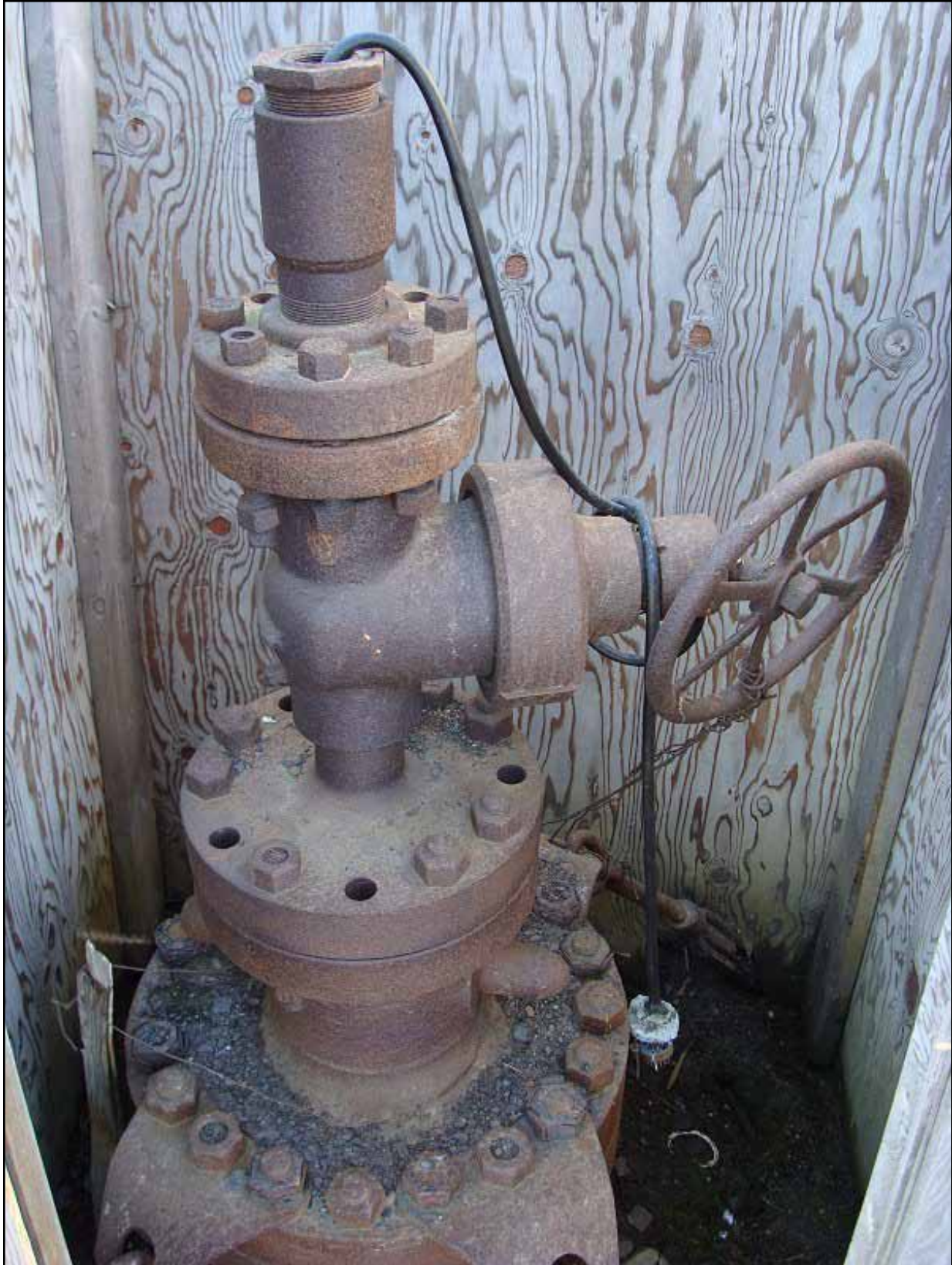
Figure 5: Wellhead for South Barrow #2; several bolts are missing on the top two flanges and the control for the gate valve still attached, but is broken. A thermistor cable protrudes from the top of the wellhead.
