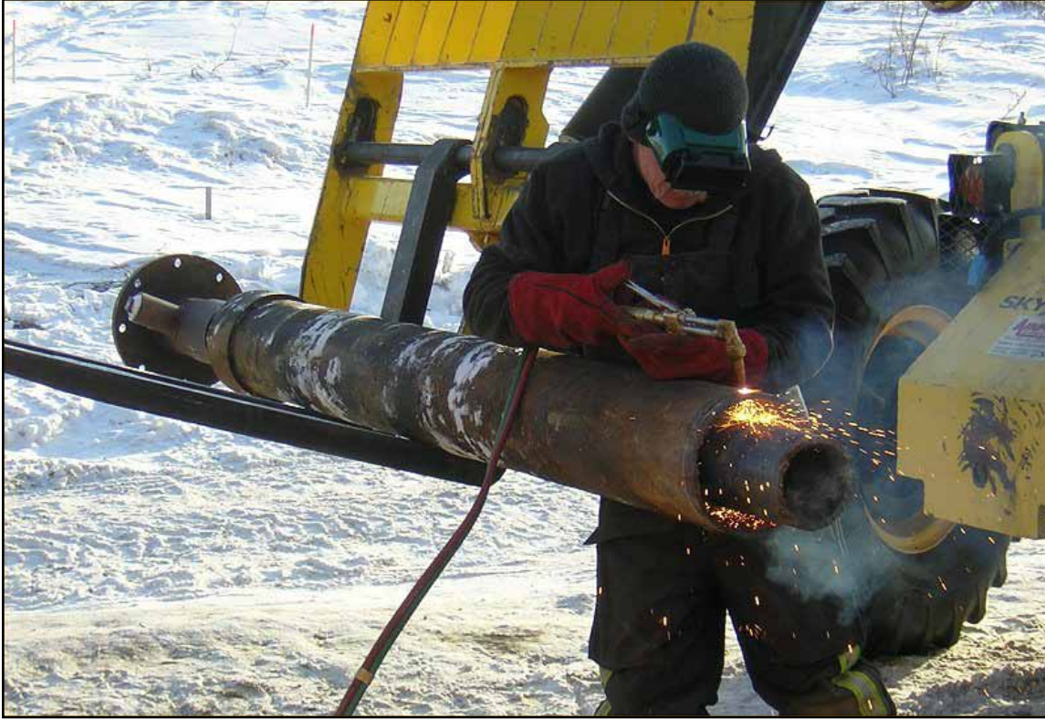
Figure 6: Cutting off the base of the wellhead casing in preparation of re-welding the wellhead to the identification plate (April 2011).
