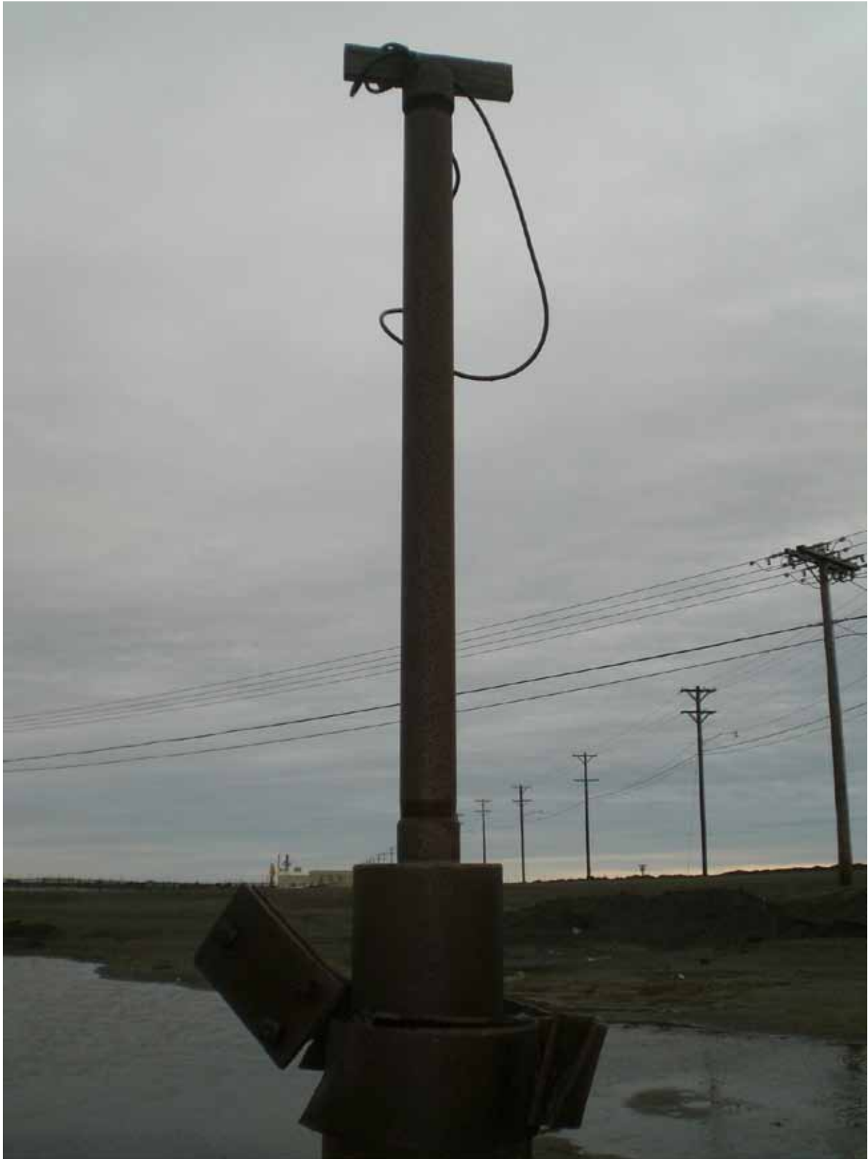
Figure 3: South Barrow #1 well close-up of pipe, note broken clamp.
