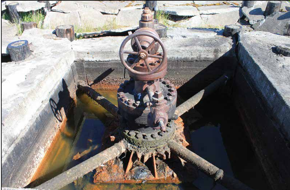
Figure 6: Fish Creek #1 wellhead with water filled concrete cellar (July 2012).
