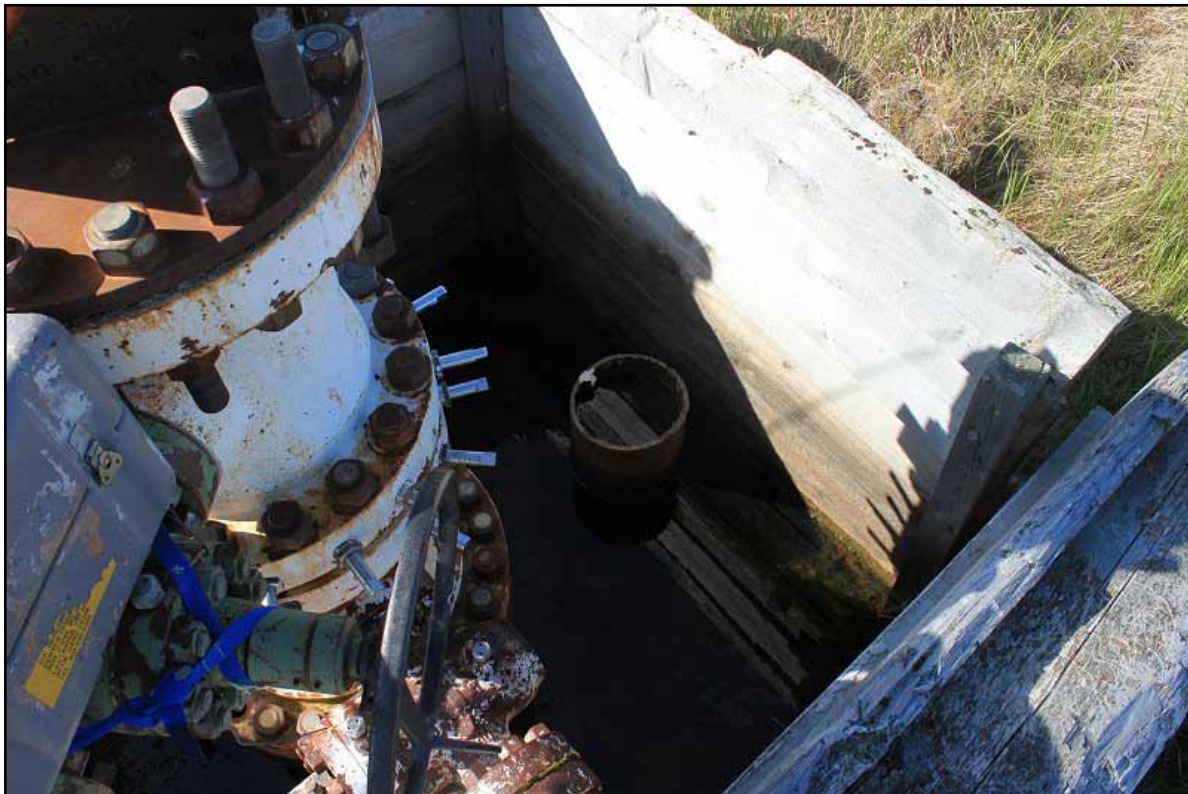
Figure 8: Rat hole inside the cellar for Kolutak #1 (July 2012).
