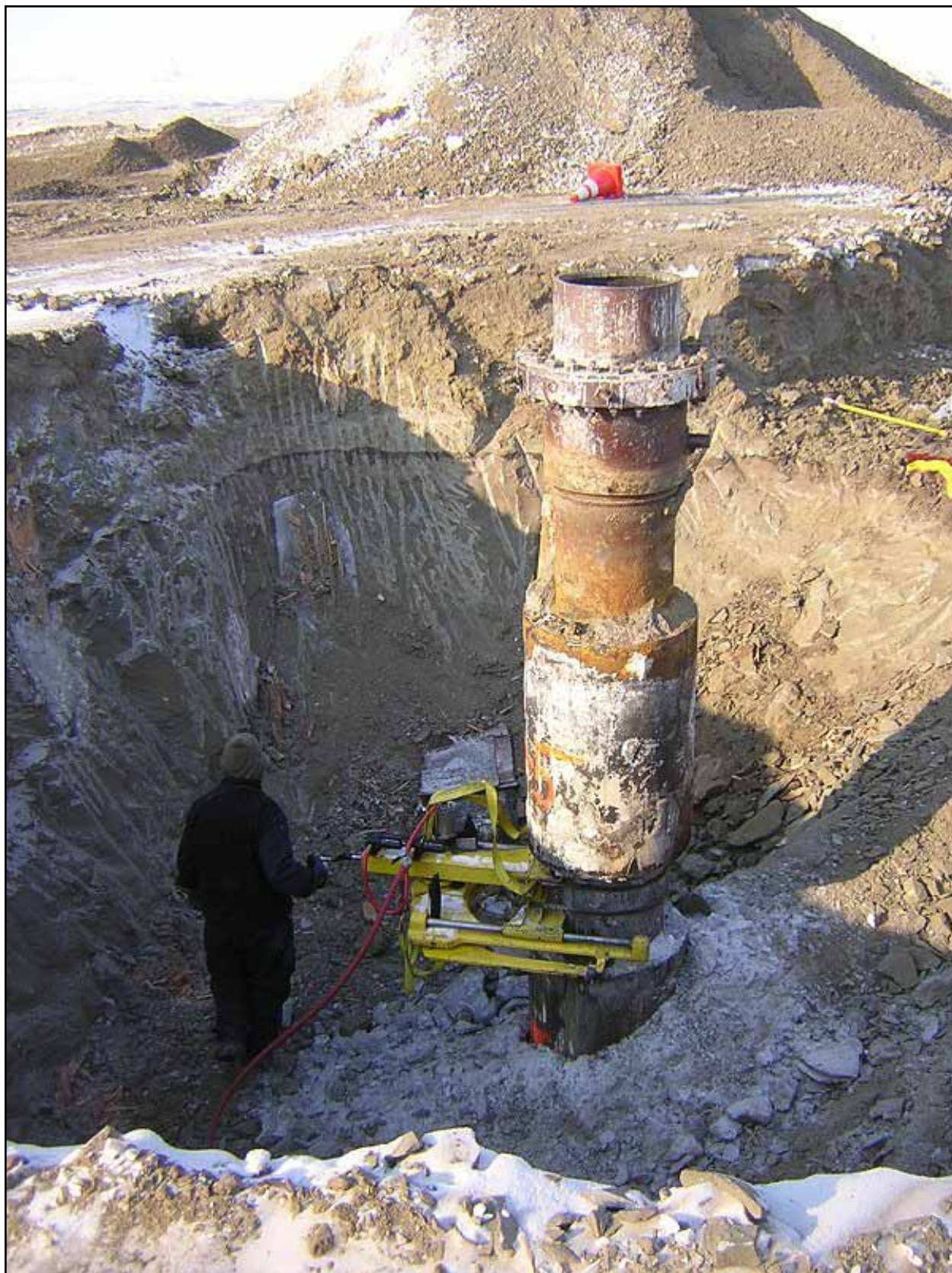
Figure 4: Removal of the Atigaru Point #1 wellbore 18 feet below the ground surface (April 2009).
