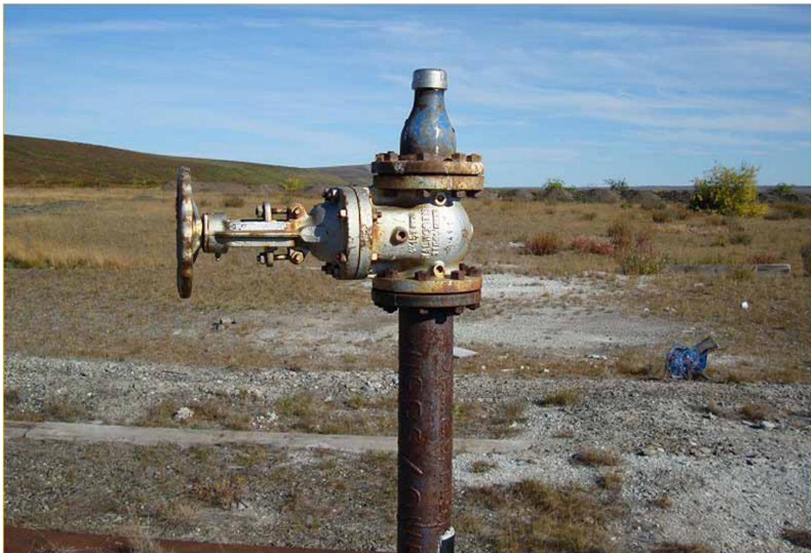
Figure 4: Gate valve on top of the line pipe at Seabee #1. This is the access point for temperature sampling by the USGS (August 2008).
