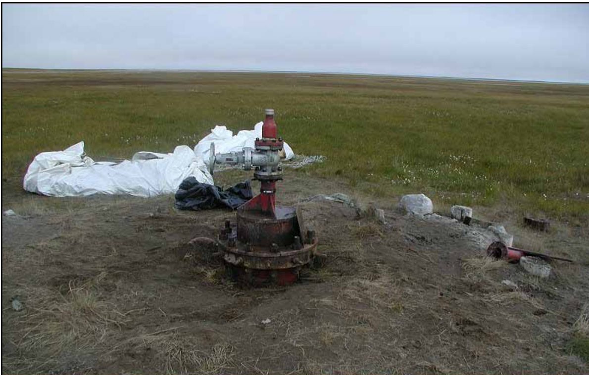
Figure 4: Installation of a new gate valve was completed at West Fish Creek #1 following the removal of the baffling and PVC downhole (August 2006).
