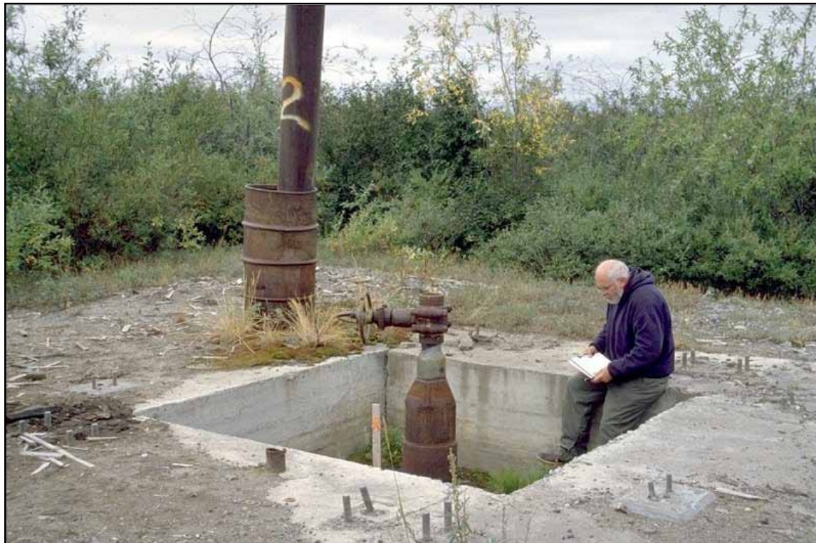
Figure 4: Umiat #2 with concrete cellar before plugging occurred (August 2000).
