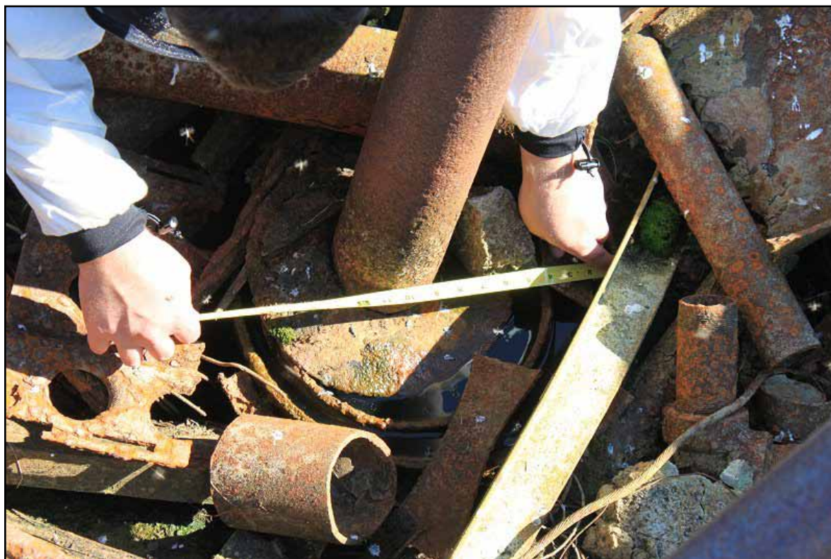
Figure 6: The 4-inch pipe is welded to a plate that covers the 11 ¾-inch casing of South Barrow #3.
