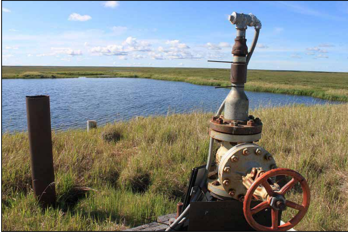
Figure 7: Functional gate valve and replaced needle valve for Kolutak #1. Temperature monitoring by the USGS occurs through the old needle valve position (July 2012).
