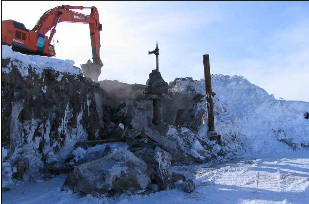
Figure 7: Excavating around the J.W. Dalton wellhead in preparation for plugging and removal of the casing (April 2005).
