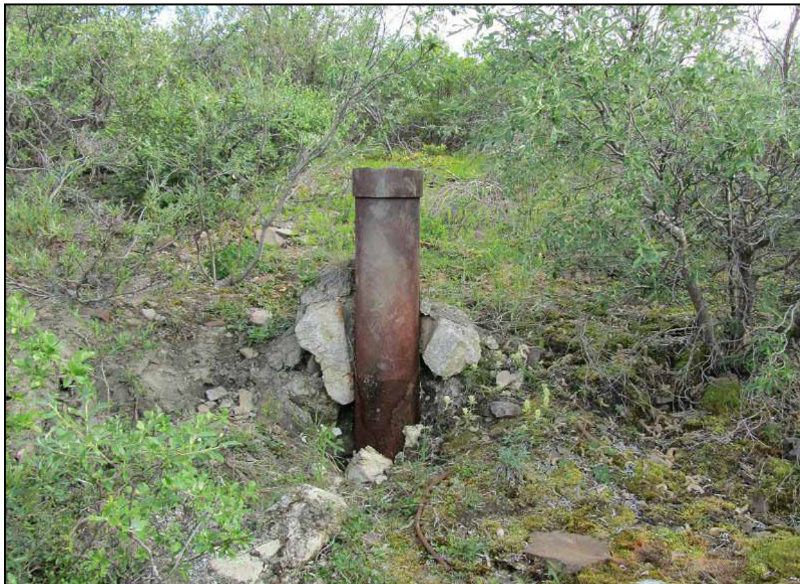
Figure 5: Knifeblade #2. showing minor corrosion occurring where the casing meets the ground surface (June 2011).
