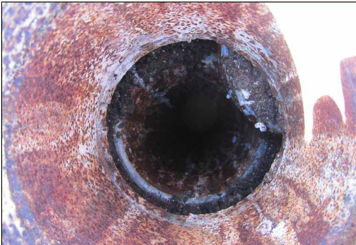
Figure 6: South Simpson #1, looking into the wellbore; the master valve is frozen in the open position.
