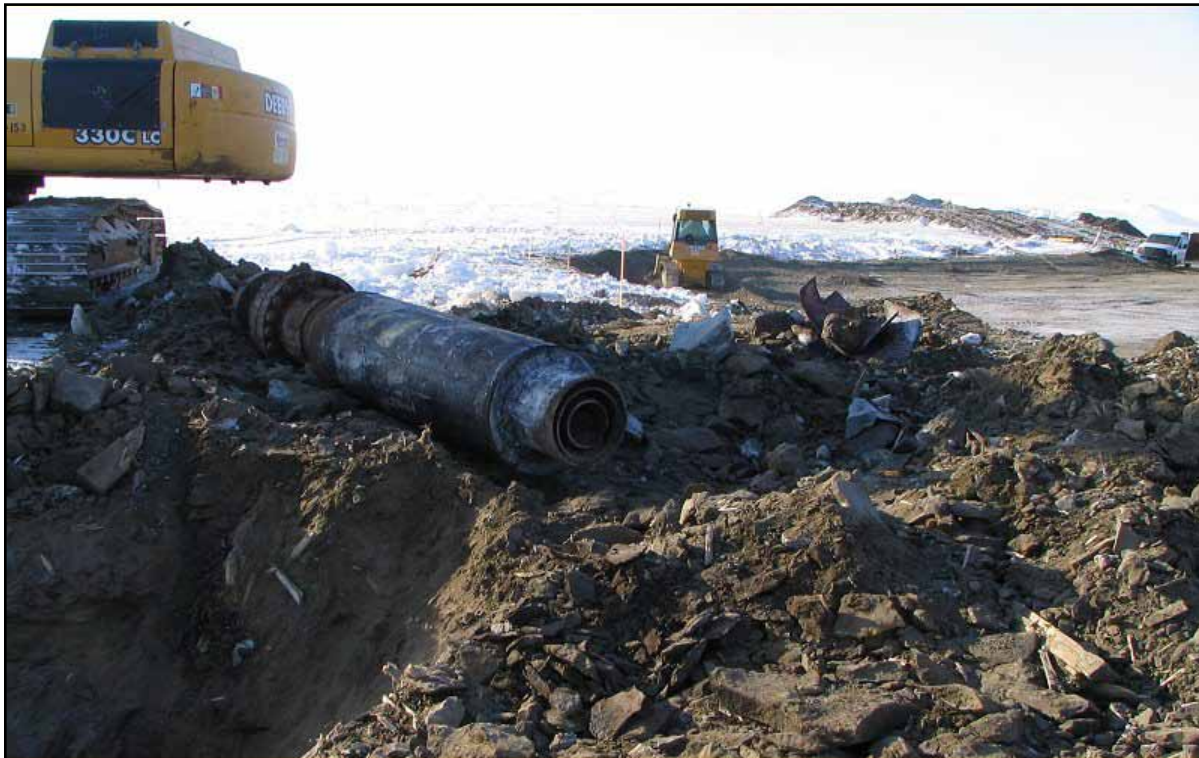
Figure 8: This shows the East Teshekpuk #1 well site shortly after cutting off the wellhead. The cut wellhead is lying next to the excavator while excavation work of the reserve pit is occurring in the background (April 2008).
