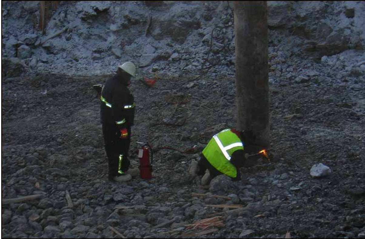
Figure 16: Cutting off the casing at 29 feet below ground level at Drew Point #1 (March 2010).
