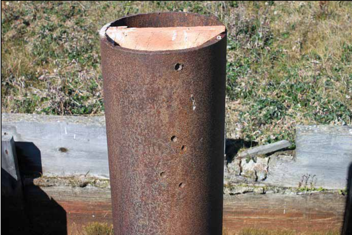
Figure 4: Close-up of Avak #1 well casing showing dents created by bullets.
