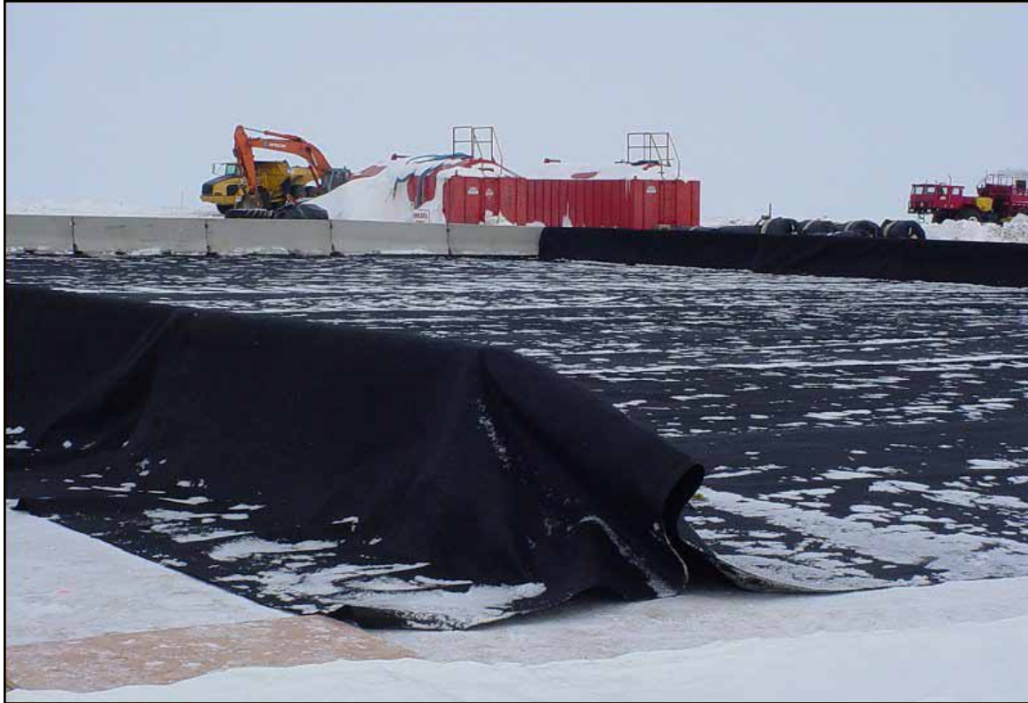
Figure 9: Lined cells created at Lonely to store excavated reserve pit material before putting in Supersacks (April 2005).
