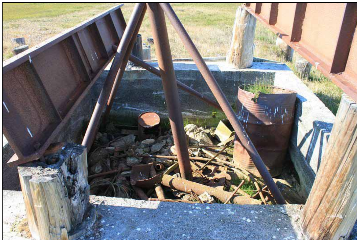
Figure 5: Close-up of debris located in the South Barrow #3 cellar.
