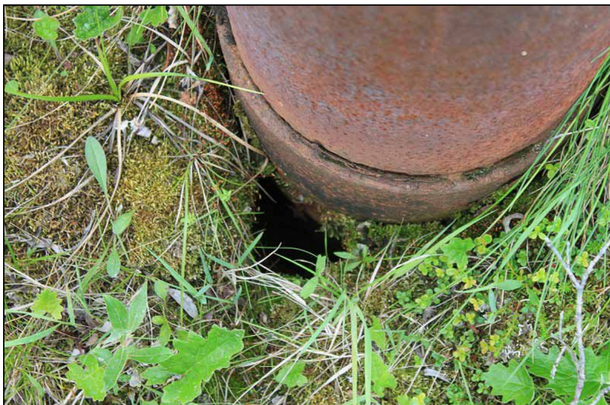
Figure 5: Ground hole around the casing at Wolf Creek #1 (July 2012).
