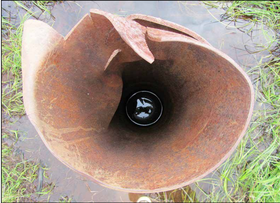
Figure 2: Knifeblade #1 damaged casing (July 2010).
