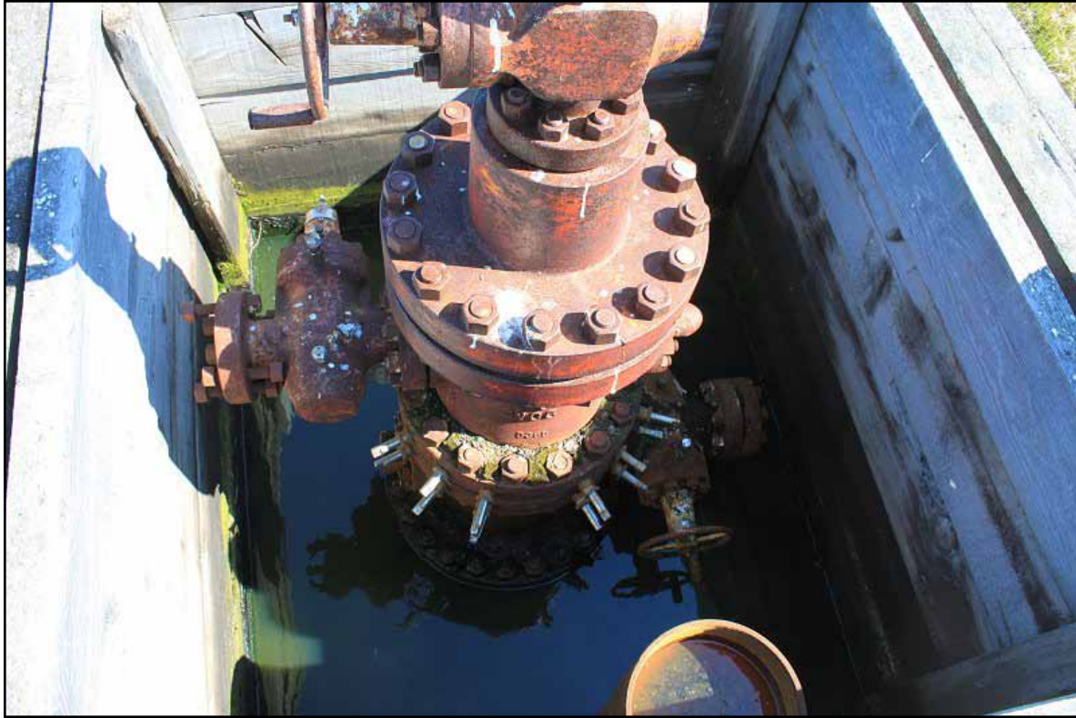
Figure 5: The Tulageak #1 rat hole is contained within the water-filled cellar (July 2012).
