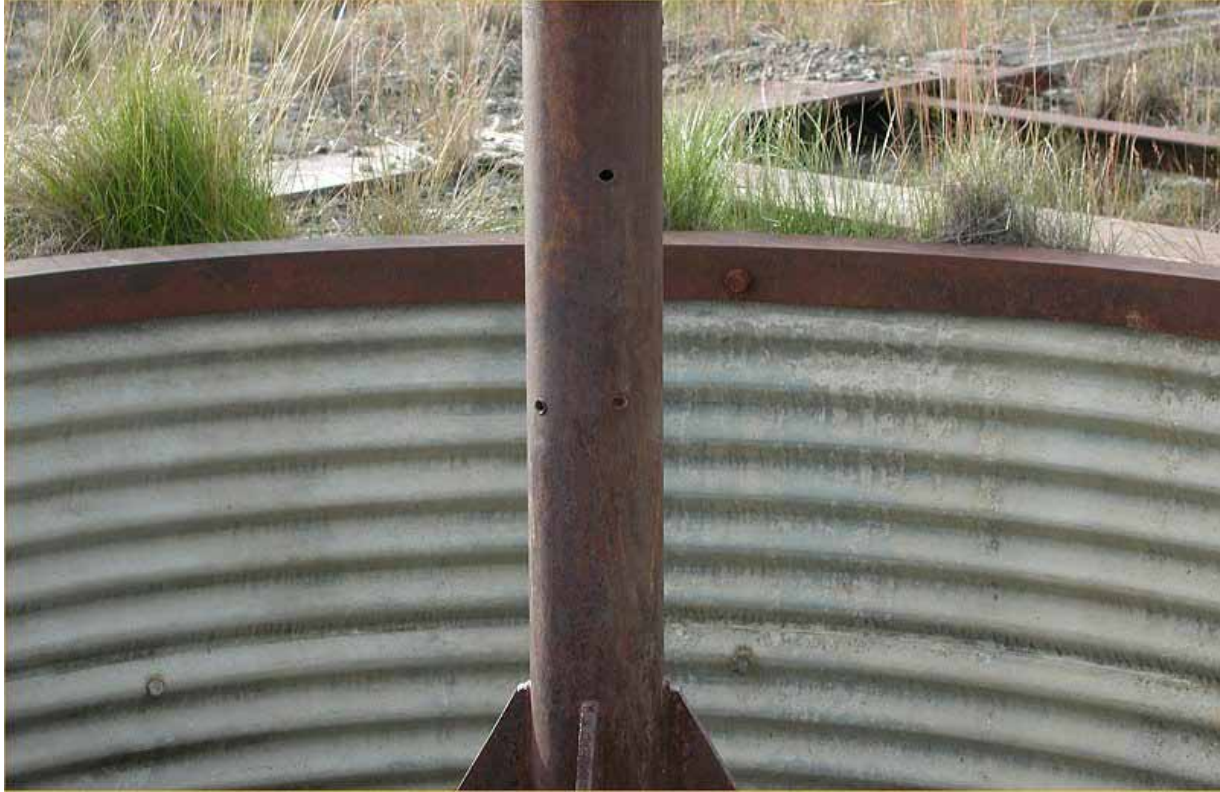
Figure 5: Puncture bullet holes in the Seabee #1 line pipe (August 2006).
