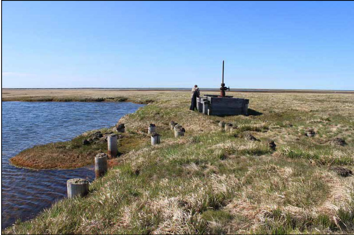
Figure 7: Tulageak #1 piling exposure along the reserve pit (July 2012).
