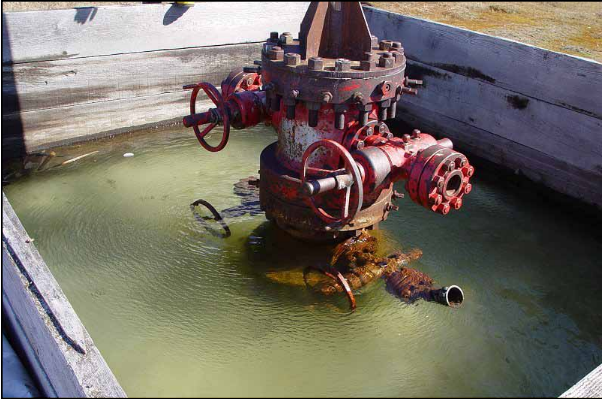
Figure 6: Cellar filled with water and wellhead at North Inigok #1 (June 2003).
