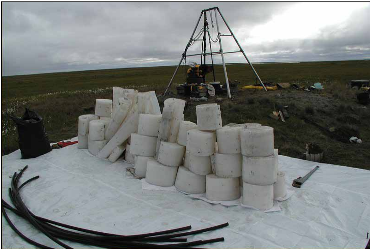
Figure 7: Extracted baffling and PVC from West Fish Creek #1 are lined up on a tarp for removal (August 2006).
