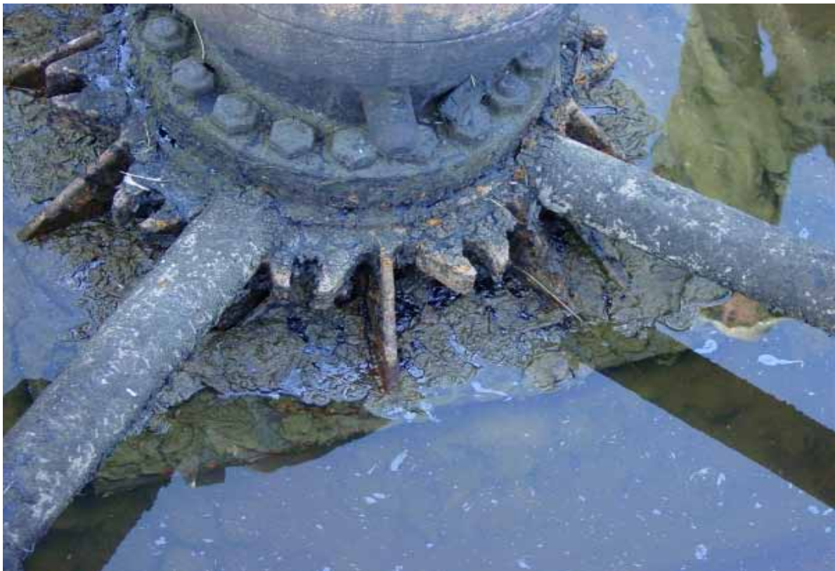
Figure 7: View inside the Fish Creek #1 concrete well cellar. Note the light sheen for the dry tar coming into contact with the cellar water. (July 2002).
