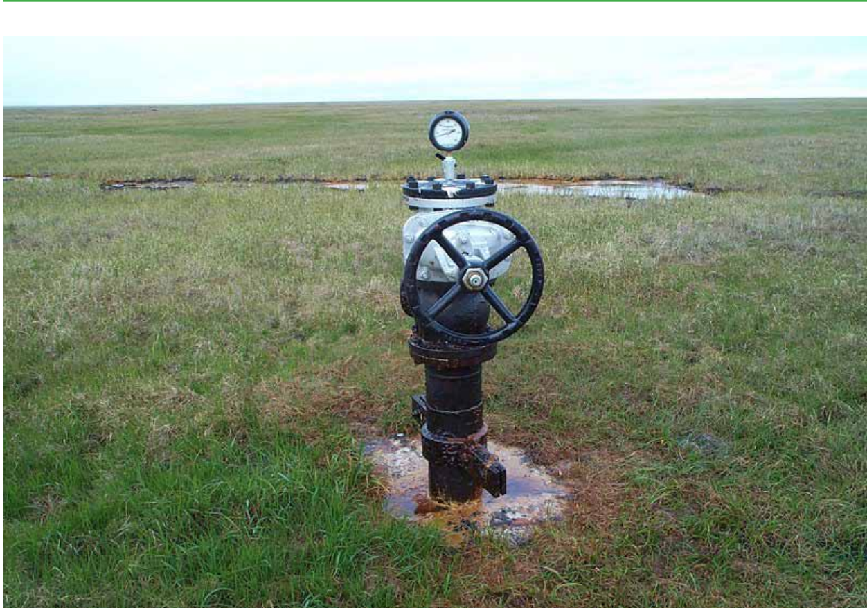
Figure 8: Simpson Core Test #31 after installing a new master valve in 2001.
