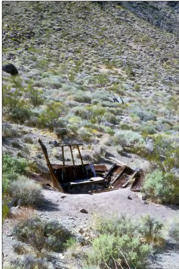
Figure 3.52. Collapsed outhouse, Leadfield, Death Valley National Park, 2000 (photograph by Karen K. Swope).
