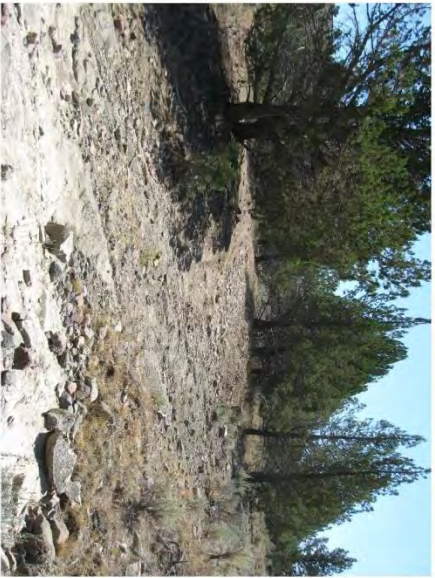
XG-24-79-S; rte around washout; Rd6263-0-AO; 7-28-09.jpg
