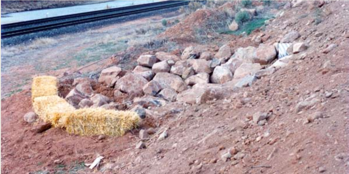
Properly sized rock rip-rap at culvert outlets helps reduce water velocity and resulting soil erosion.
