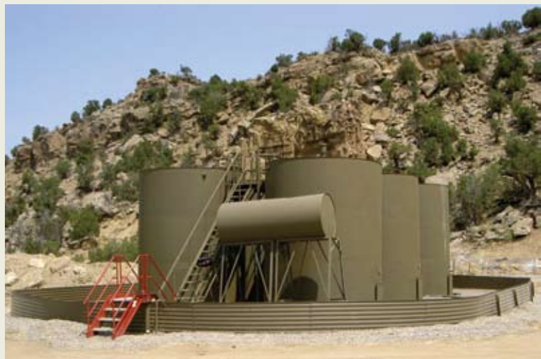
This central tank battery has been surrounded with a corrugated metal containment wall.
