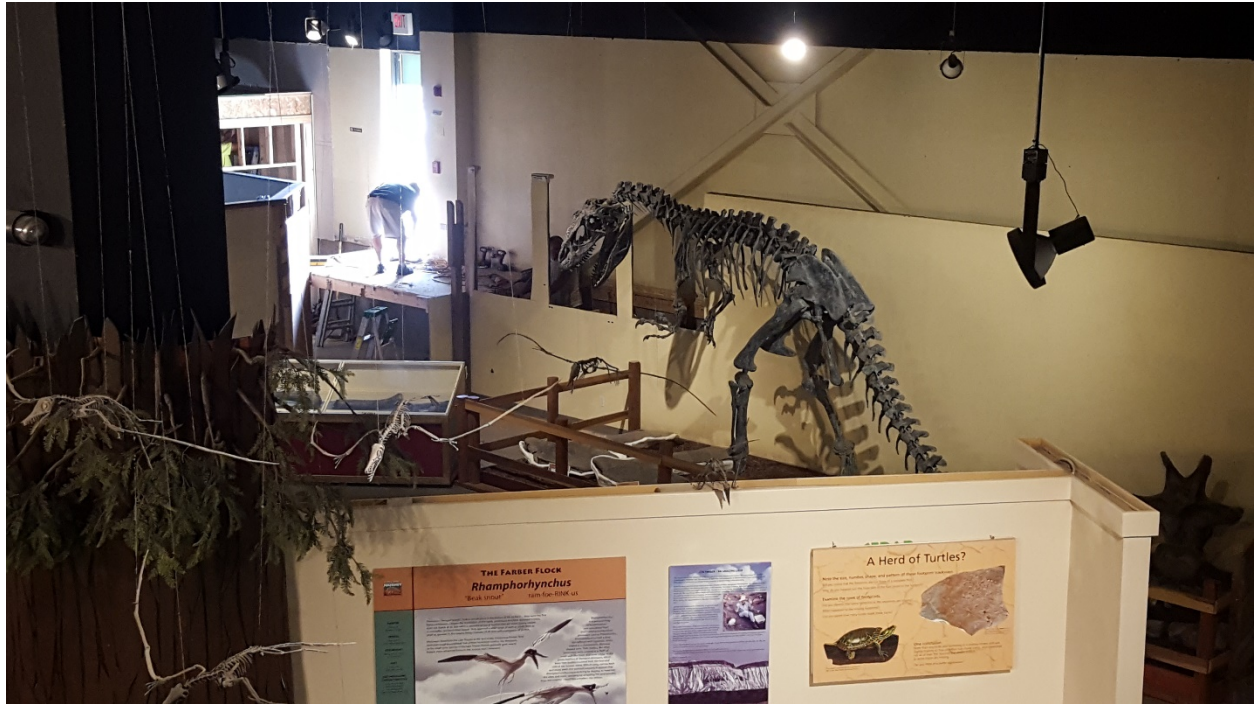
Removing the exterior door and walkway behind the Allosuaras exhibit at Dinosaur Journey museum.
