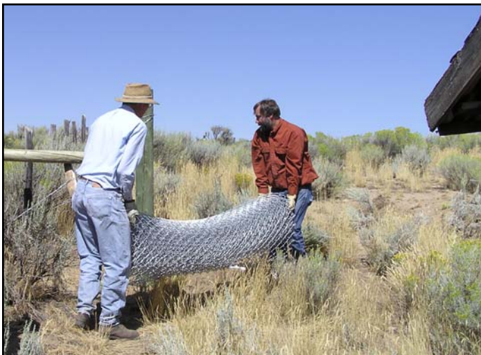
BLM employees Mike Jensen and Frank Blomquist carry galvanized fence. Fencing off old buildings was an important first step to the long-term vision for the historic property.
