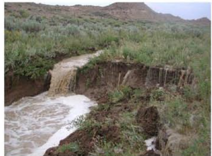
NATURAL DRAINAGE FLOODING AND DOWN-CUTTING AS A RESULT OF STORM RUNOFF. NOTE: SURFACE RUNOFF AND PIPING ON EDGE OF THE HEADCUT.
