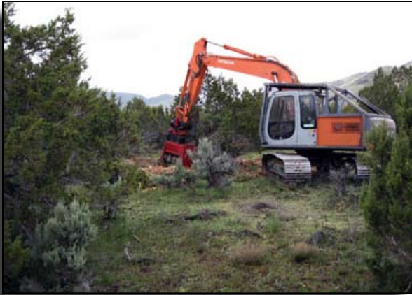
Mastication equipment is used on private land in Elba, Idaho, to help reduce the threat of wildfire for homeowners. Mechanical treatment such as this is safer than prescribed burning in this wildland urban interface area.
