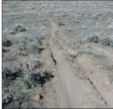
Use during wet conditions has negatively affected adjacent natural resources.
