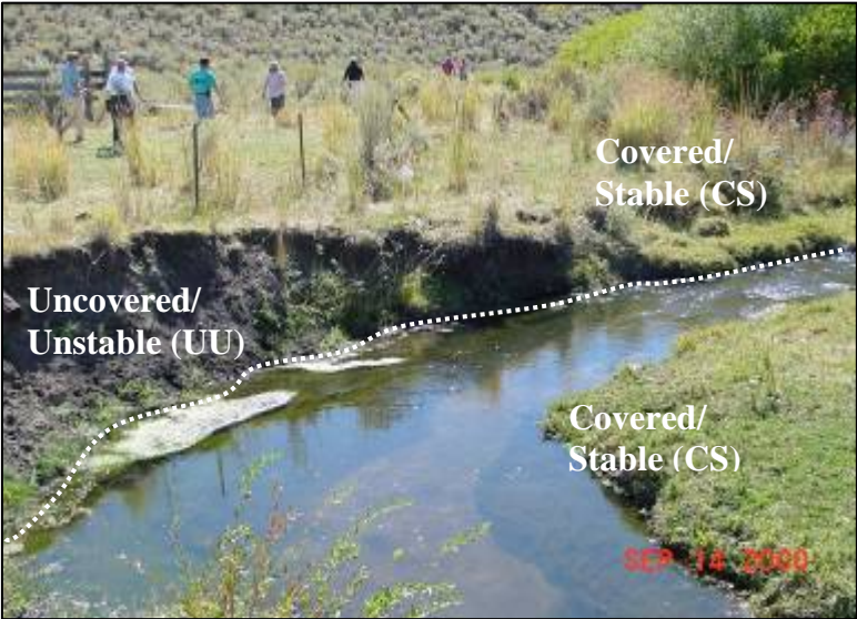
Figure 12 —the scour line is near the current water level. The streambank classification reflects the bank from scour line to first terrace. The bar is covered, therefore stable.
