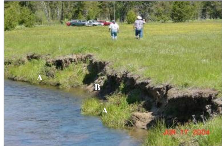
Figure 6 —the stream in this photo is flowing at the scour line. Slumps “A” are still attached to the bank above the scour line and would be classified as covered/unstable (CU) (see Illustration 4). “B” has no vegetation along the streambank and is uncovered/unstable (UU) (see Illustration 3).
