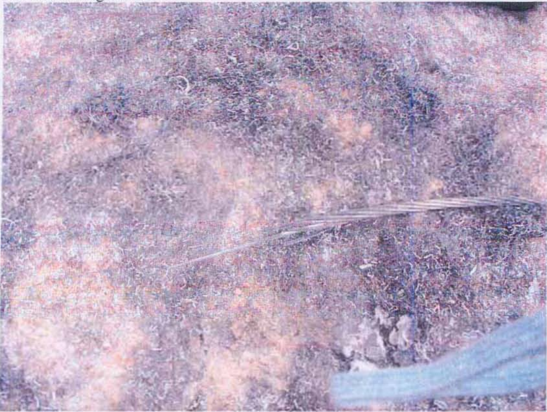
Photo # 11 Same end of power line shown in photo #10, laying on the ground.
