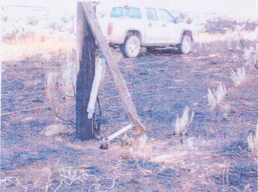
Photo # 8 Closest power pole where line went down. Note: broken power line on the ground to the right of pole. Facing South West.
