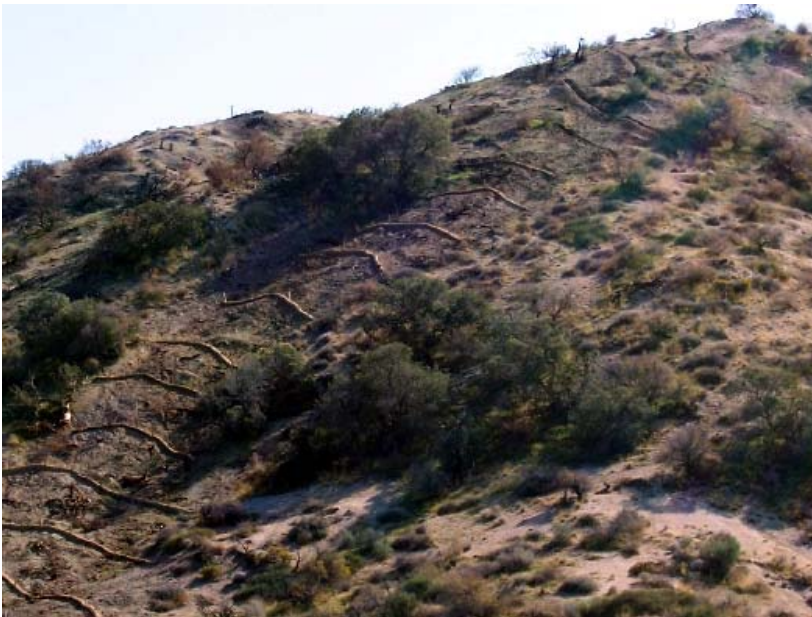
Straw wattles installed on a large dozer line slope to control erosion, Big Morongo ACEC.
