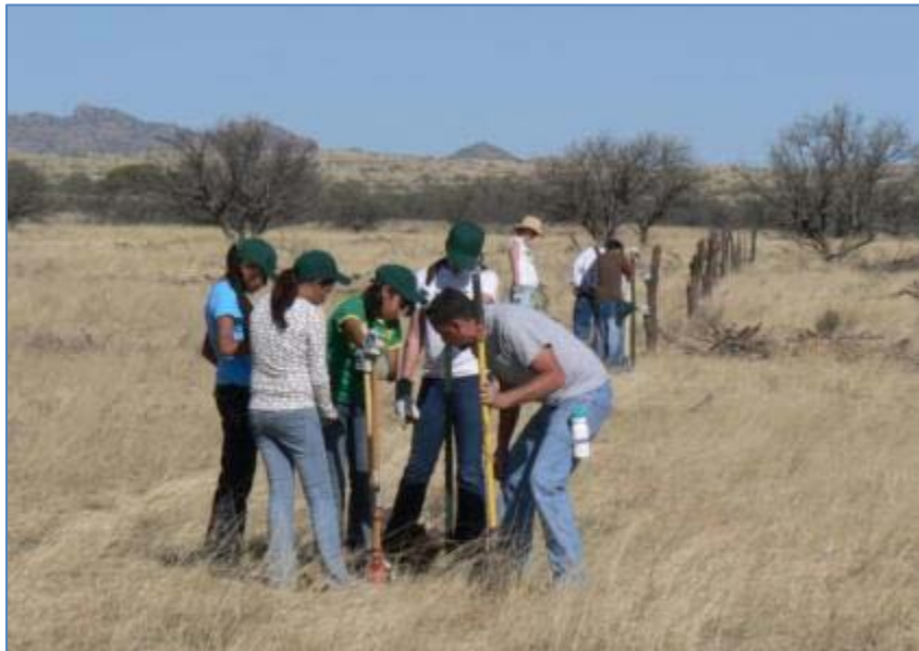
Figure 19- Hohokam Middle School students installing fencing at a group recreation site on LCNCA
