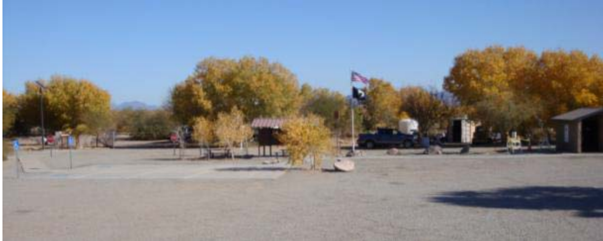
Photo 2: A new concrete parking area and walkways at the Oxbow Recreation and Wildlife Area provide universal access to restrooms and the boat launch.
